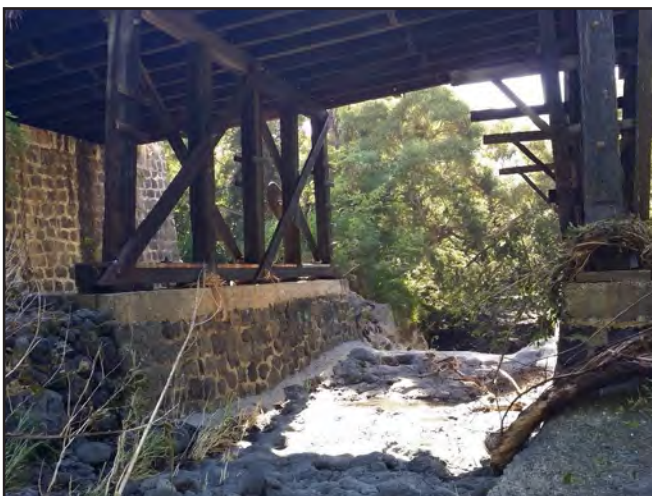
Photo 3. Ninole Bridge timber columns and footings on mauka side of bridge, view downstream
