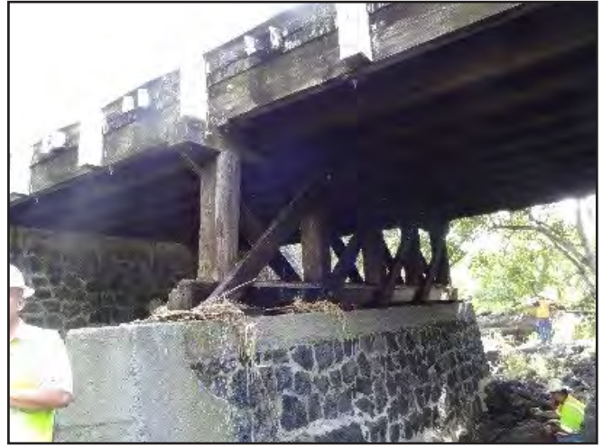
Photo 2. Hilea Bridge timber columns and footings on makai side of bridge, view upstream
