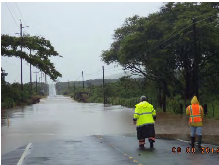
Photo 3-2b. Overtopping of roadway northeast of Hilea Bridge during Tropical Storm Iselle.
