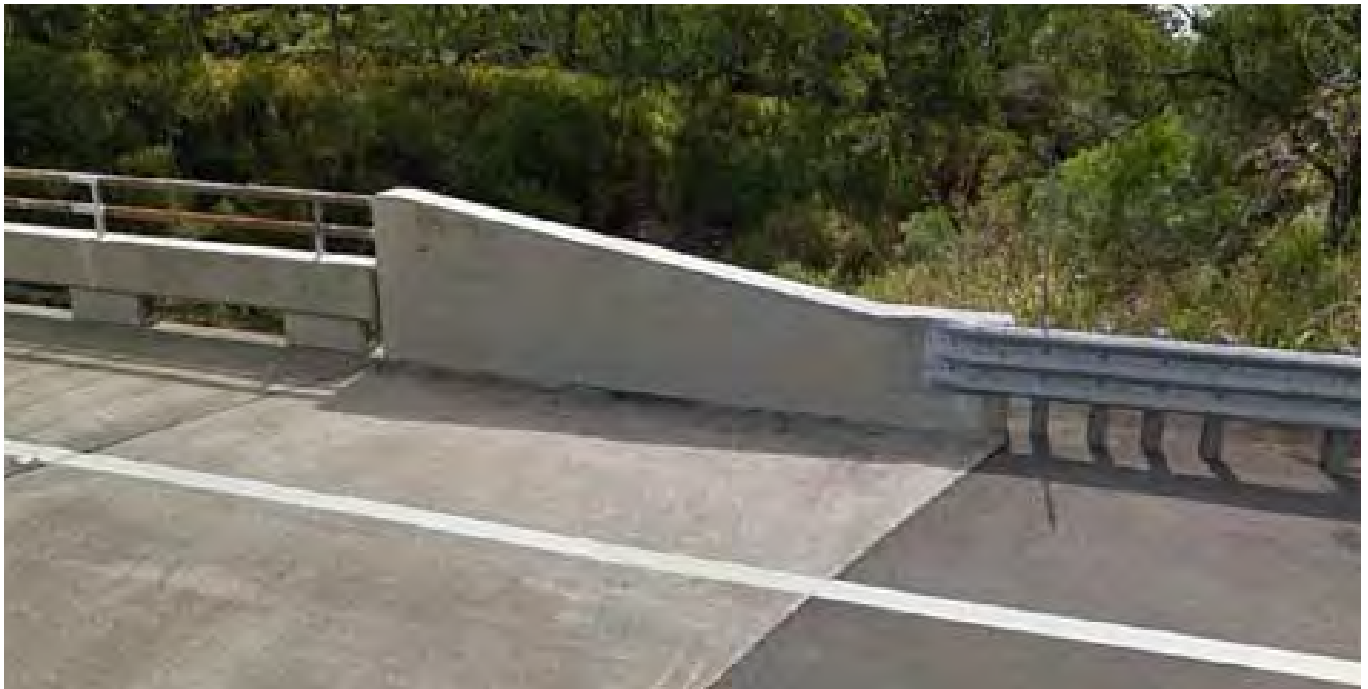
Representative bridge railings on the Keaiwa Stream Bridge, located at Mile Post 50.35, approximately 6-7 miles from the Hilea and Ninole Bridges.
