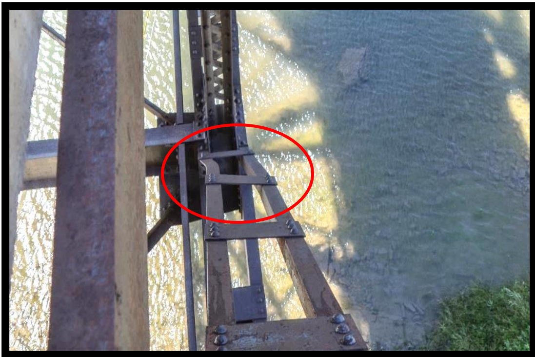
Photo 10 – Member U5B to L4B. Note buckling of member.
