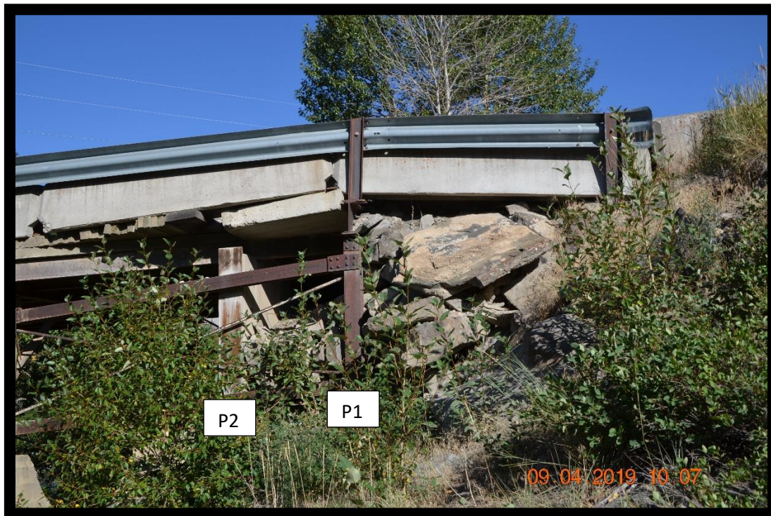
Photo 14 – Downstream Face of Left Abutment. The slope debris behind P2 is producing considerable lateral load to P2 and P1 that could lead to failure of the left abutment approach span. Note concrete jersey barriers leaning on steel guardrails.
