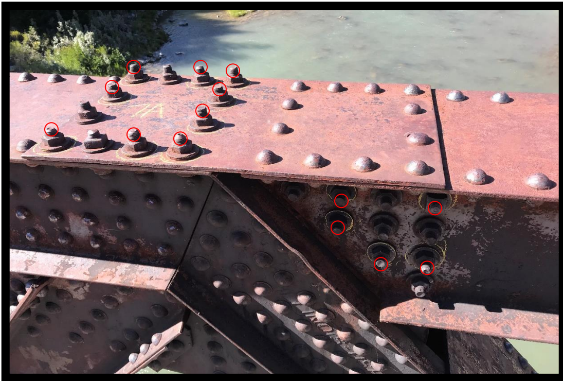
Photo 13 – Looking Upstream at U7A From Bridge Deck. 14 bolts were observed to be loose. Marked in the field with yellow crayon but circled red here for clarity.
