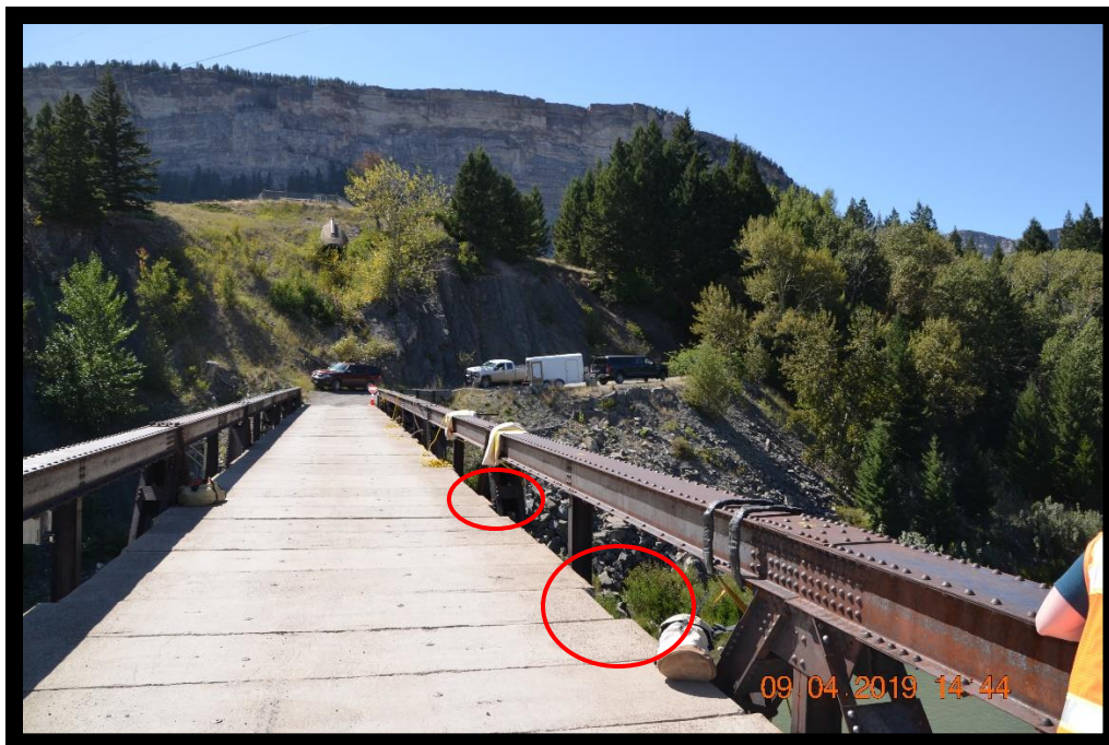
Photo 8 – Bridge Deck Looking Towards Right Abutment. Note laterally offset concrete deck planks because they are not restrained to the stringers. Also note sharp, narrow approach in background.
