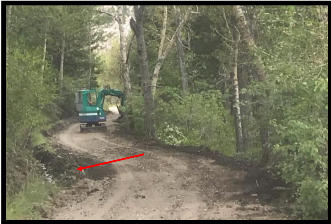
Photo 5 – South Approach Road. Photo shows regular maintenance by mini-excavator needed to clean ditches and redirect seepage losses from the Pishkun Supply Canal. Regular excavator or backhoe is too large to do work. Lining the PSC would eliminate the groundwater issues and geotechnical concerns.
