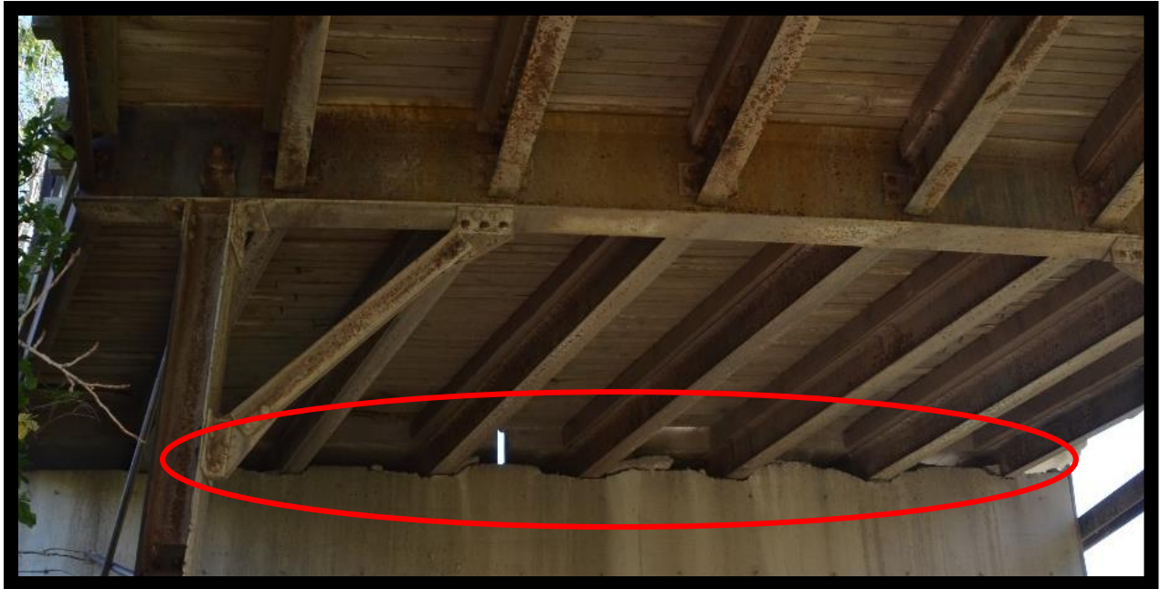
Photo 9 – Left Abutment Backwall. Note the concrete is being crushed where the stringers brace the left abutment backwall.
