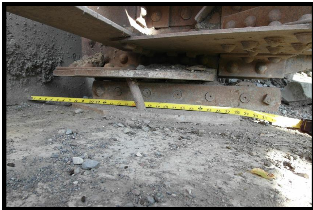
Photo 6 – Right Abutment Roller Bearing System. Note right roller is off the bearing plate and bent anchor rod is sheared at the top of the plate.
