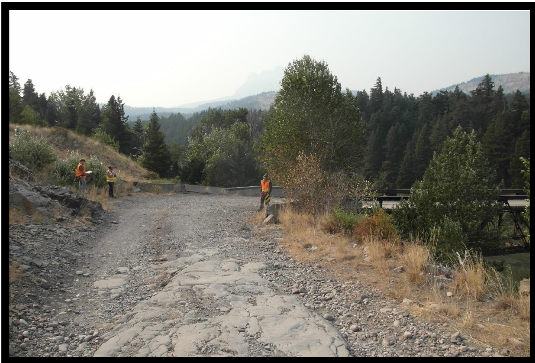
Photo 4 – Left Bridge Abutment. Note right angle turn onto bridge and exposed bedrock in approach subgrade.
