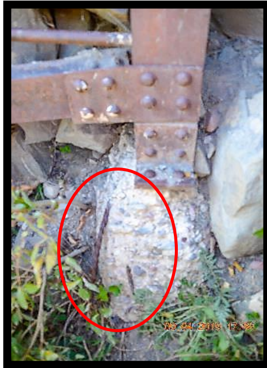
Photo 7 – Approach Pier (P1) on Downstream Face of Left Abutment. Note deteriorated concrete and exposed rebar.
