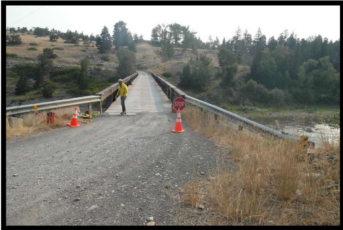
Photo 3 – Right Bridge Abutment. Note narrow and crossing sharp curves on the approaches.
