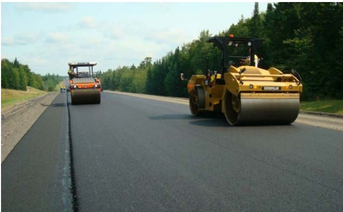
Double drum steel wheel vibratory roller machines smooth a newly paved roadway. Photo courtesy of Transtec, Inc.
