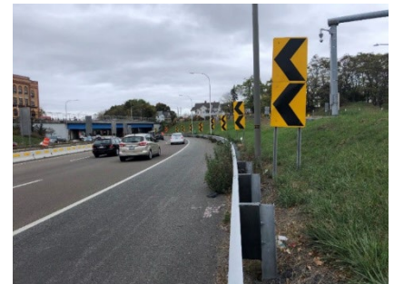
High friction surface treatment, guardrail, and enhanced signage at I-95 northbound Pawtucket S-Curve, Pawtucket, Rhode Island. (Source: FHWA)
