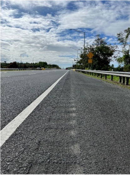
Shoulder rumble strips in Puerto Rico. (Source: FHWA)
