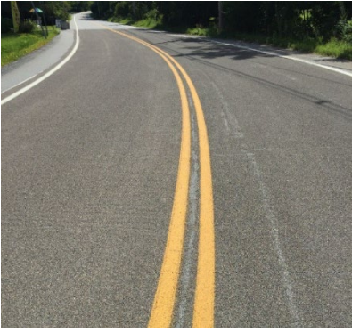
High friction surface treatment at Mossup Valley Road, Foster, Rhode Island. (Source: FHWA)
