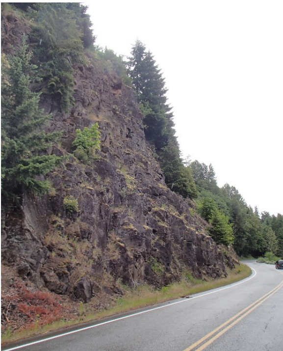
Figure 18. Rock cut where failure is controlled by interaction between geologic structure and rock friction. Forest Service Road 90, Milepost 13.
