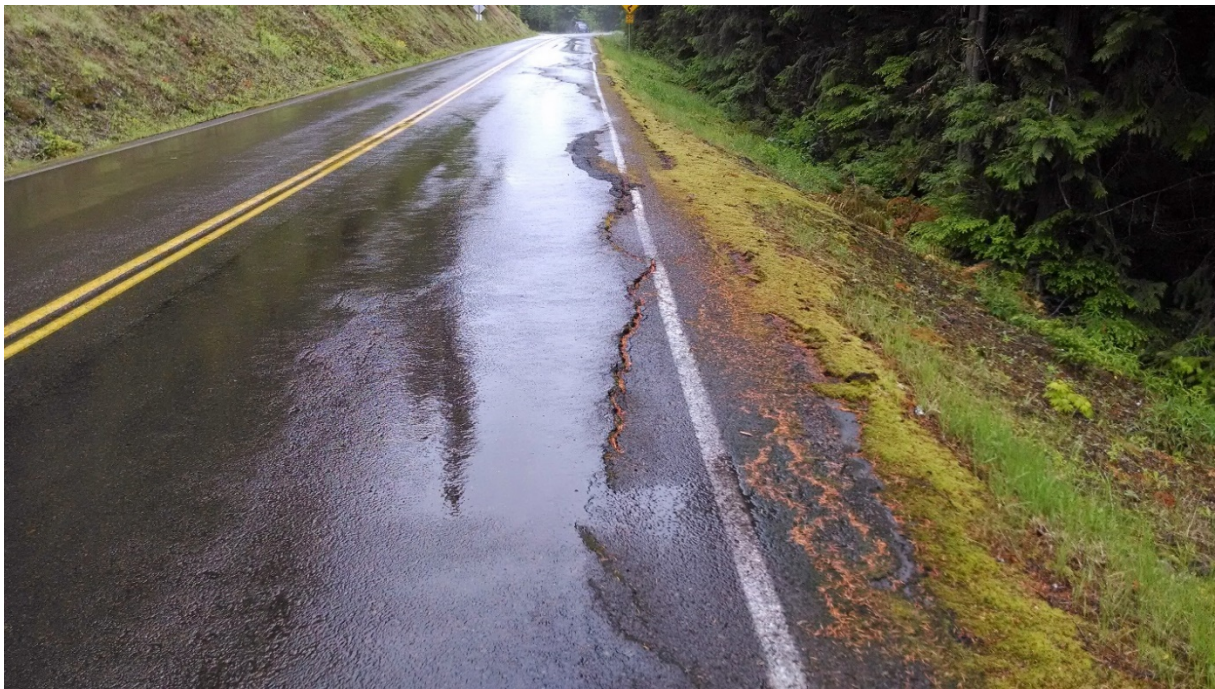
Figure 5. Embankment failure affecting up to 25 percent of the roadway. Forest Service Road 25, Milepost 30.
