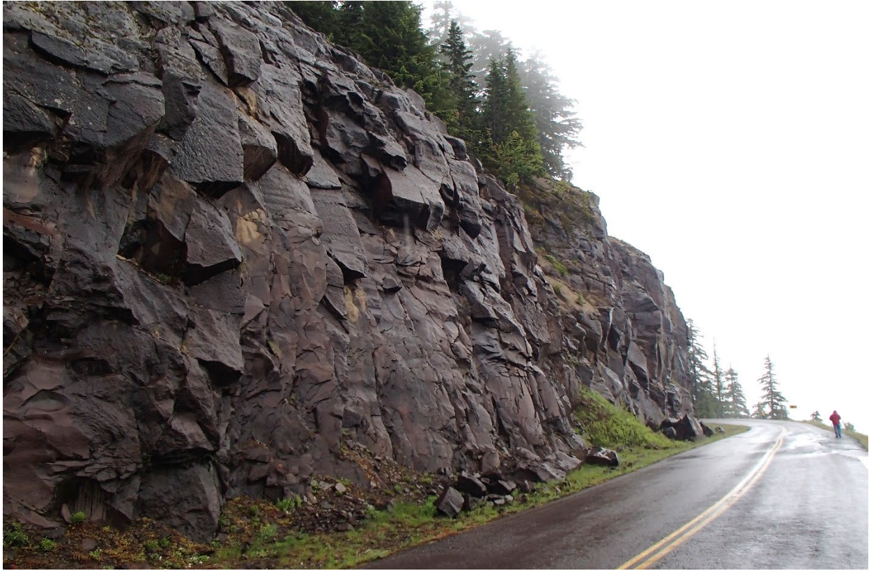
Figure 10. Rockfall debris in the roadside ditch can be used to help assess both block size/event volume and failure type. Forest Service Rd 25, Milepost 25.
