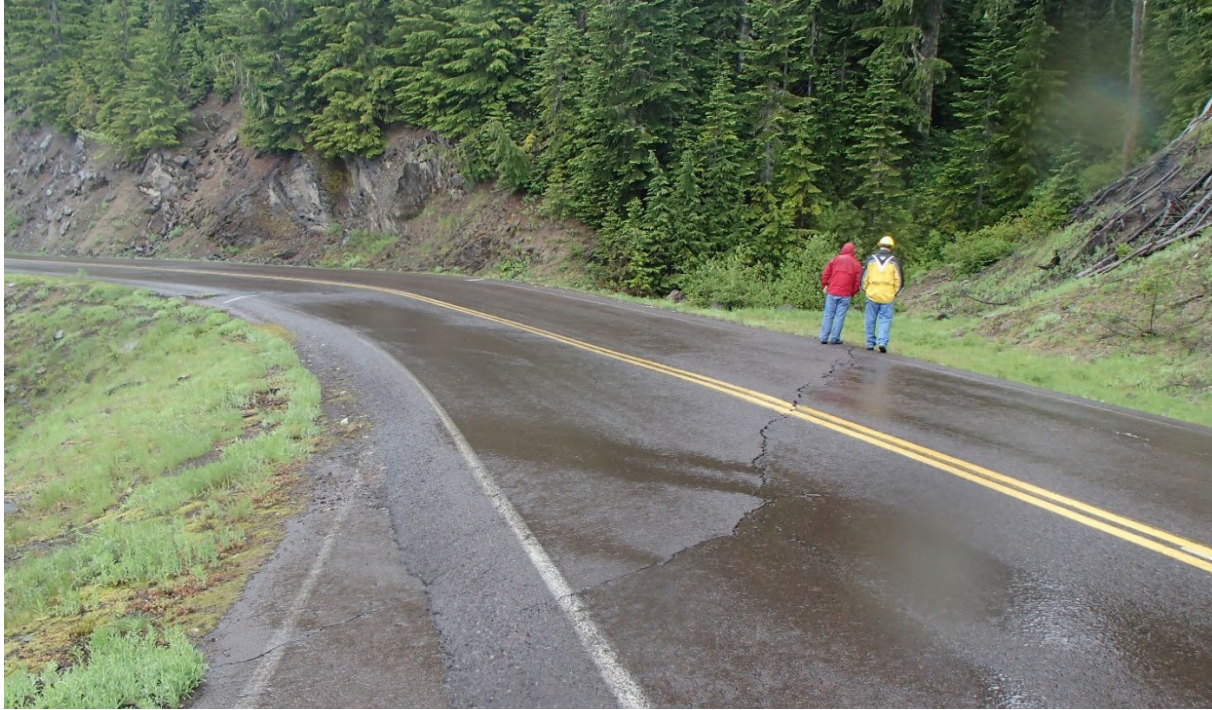
Figure 6. Embankment failure affecting entire roadway. Forest Service Road 25, Milepost 25.
