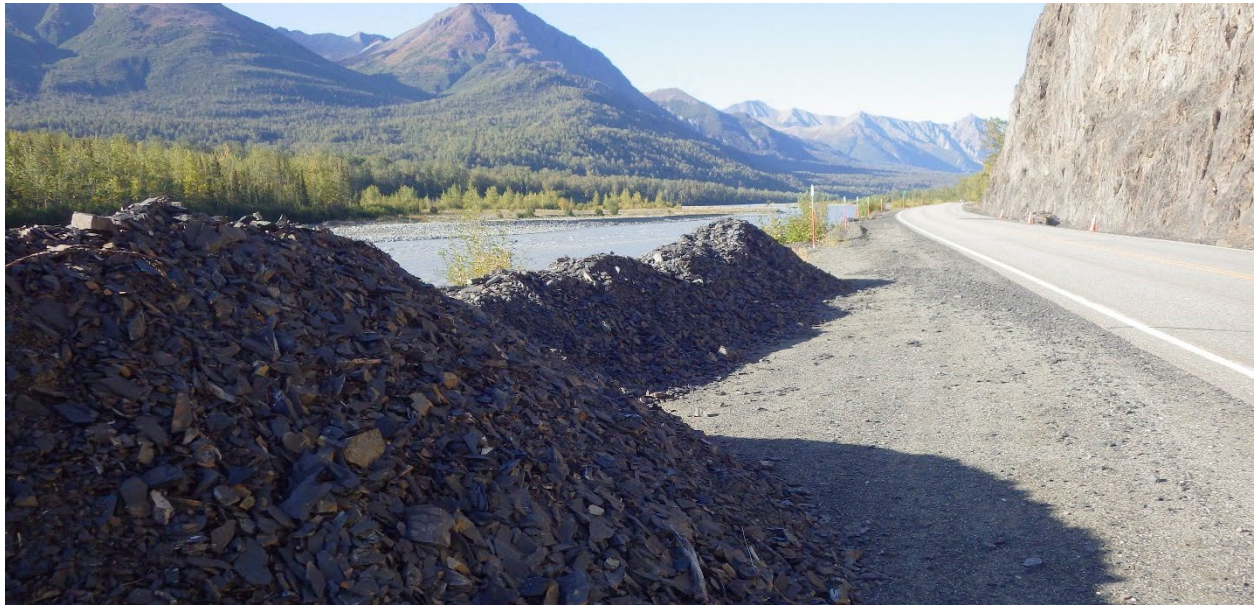
Figure 17. Constant rockfalls occur at this rock slope on the Glenn Highway in Alaska. Maintenance personnel stockpile the daily debris in this pullout for regular removal. This rock cut received a category score of 81.
