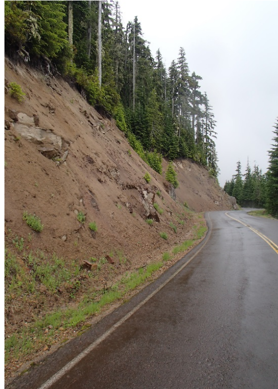
Figure 20. Rock cut where differential erosion is the dominant cause of failure. Forest Service Road 25, Milepost 30.
