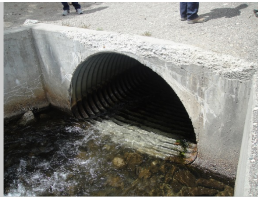
Inlet Headwall – Note deteriorated concrete
