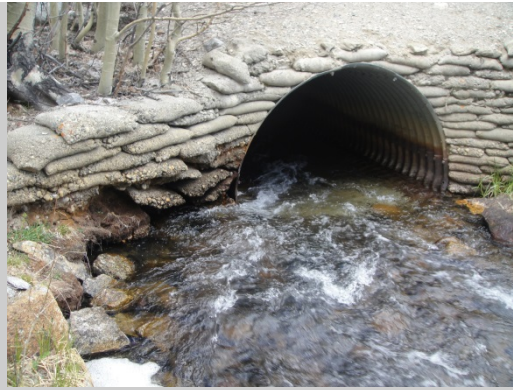
Inlet – Note undermining of the wingwall
