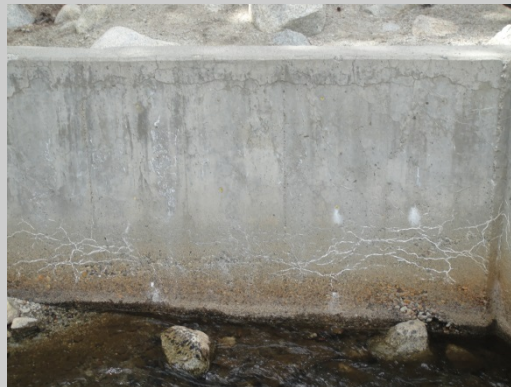
Inlet Wingwall – Note condition of concrete
