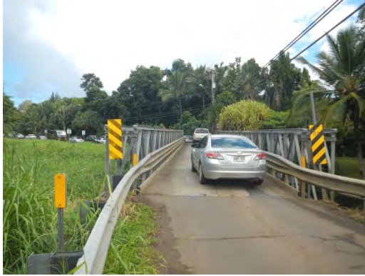
Pavement conditions near Bridge 2
