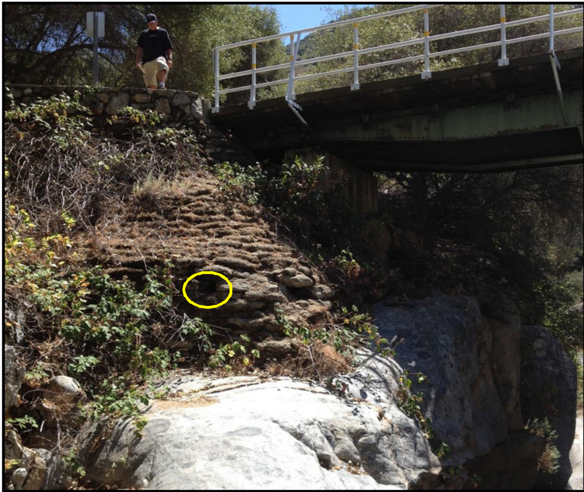
Photo #11 – Void in Cement Bag Wall (Abutment 2)
