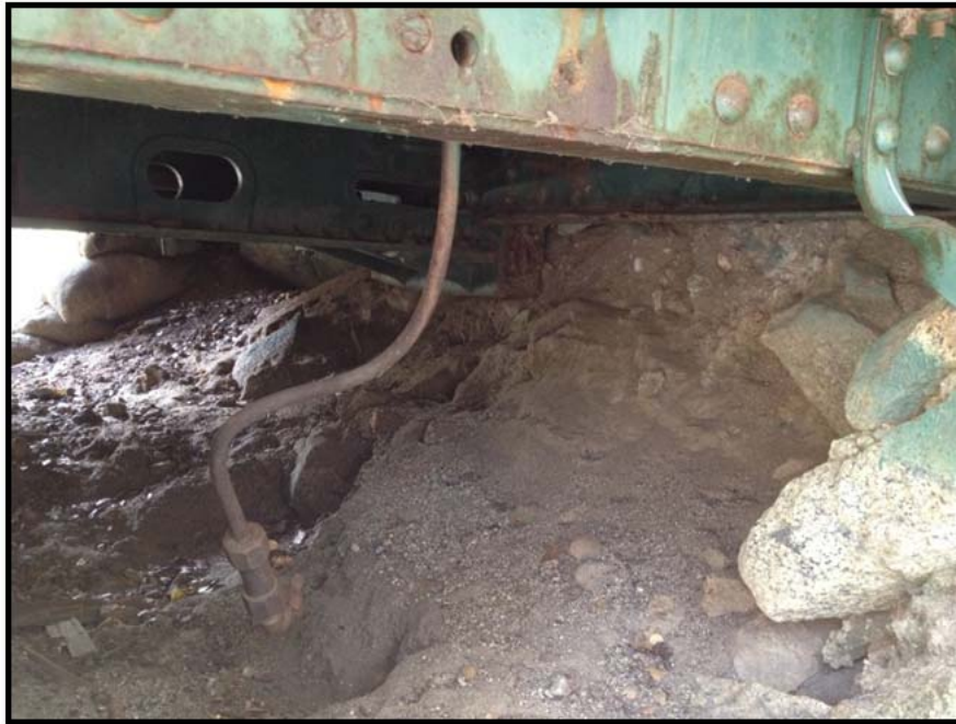
Photo #7 – Erosion at Abutment 2
