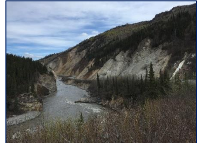
The highway is constrained by areas of slope instability and erosion by the river in the Nenana Canyon (MP 239-241)
