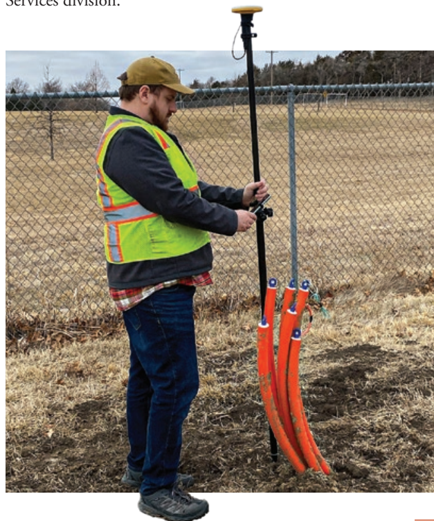
Linear construction projects, including this fiber-optic conduit system, were undertaken as part of the pilot project. © 2024 Braeden Beck / JEO Consulting Group.
