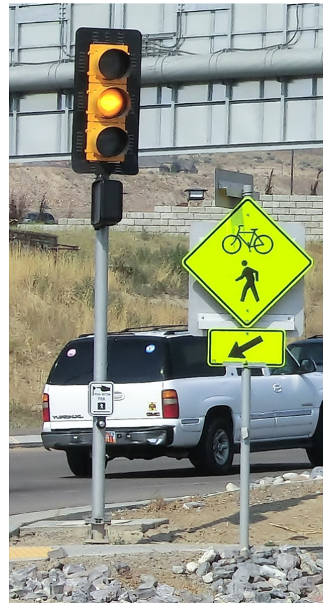
Appropriately timed yellow change intervals can reduce red-light running and improve overall intersection safety. Source: FHWA
