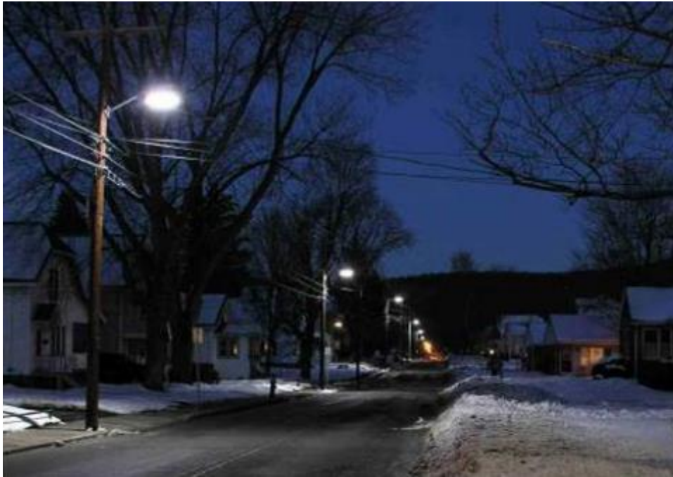
Utility poles with attached street lighting fixtures placed with a lateral offset from the road curb.
