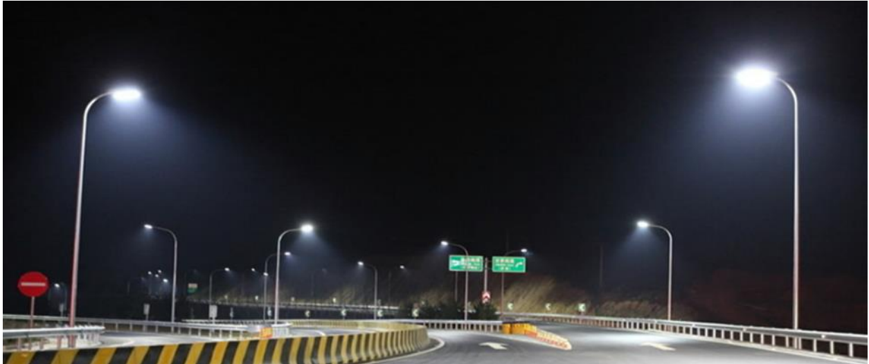
Potentially glaring luminaires along a highway at night.
