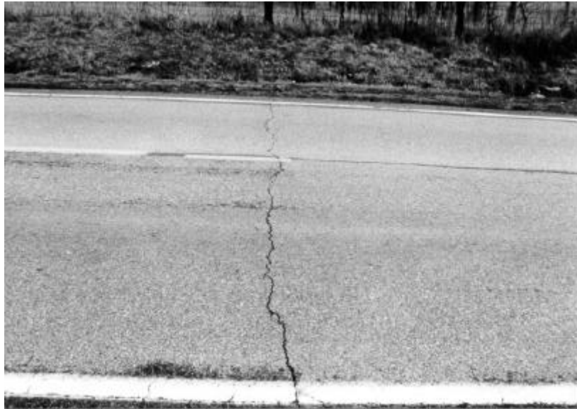
Figure 4. Pavement candidate for transverse crack sealing.
