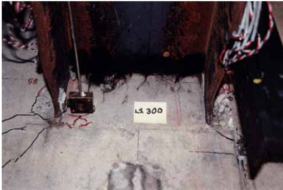
Figure 3-31. Local buckling of steel-pile flange at the conclusion of testing.
