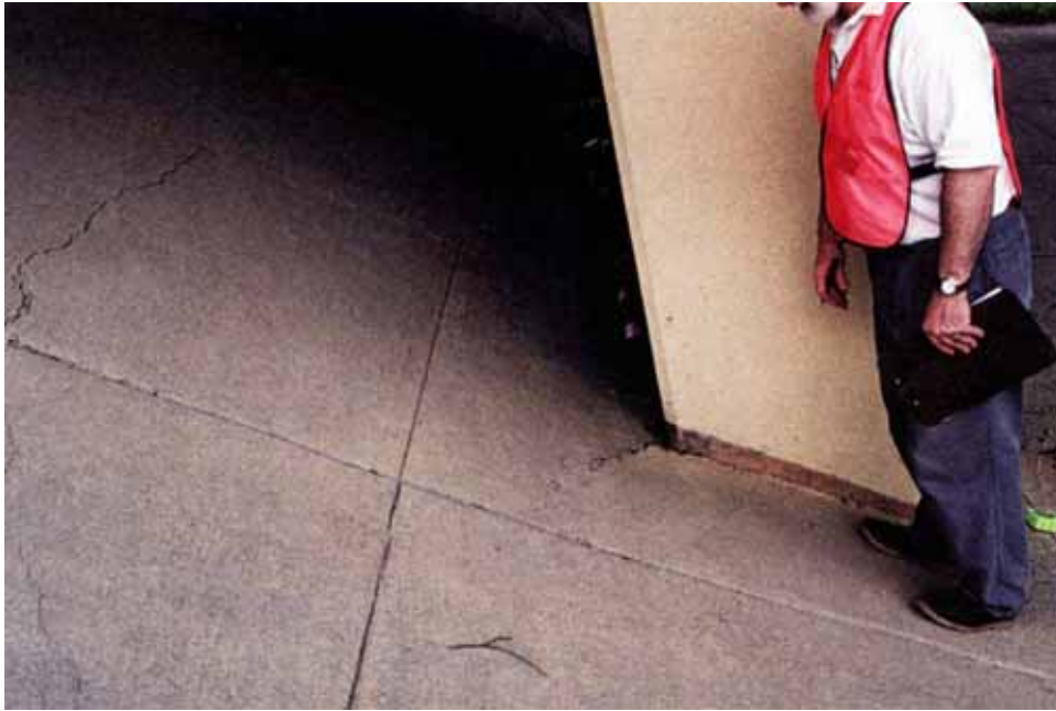
Figure 3-42. Bridge 10—cracking in slope pavement.
