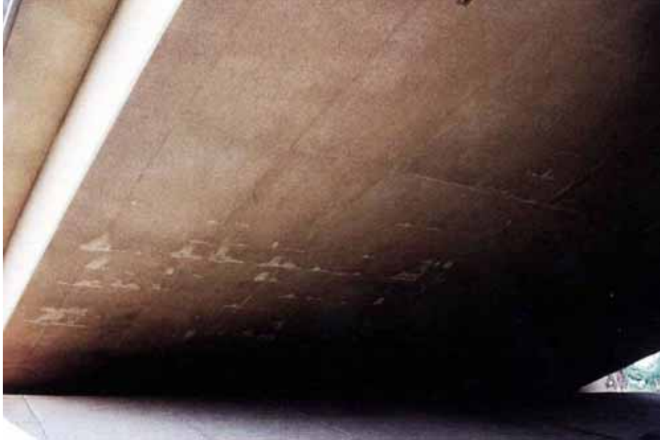
Figure 3-37. Bridge 10—cracking in bottom flange near north abutment.
