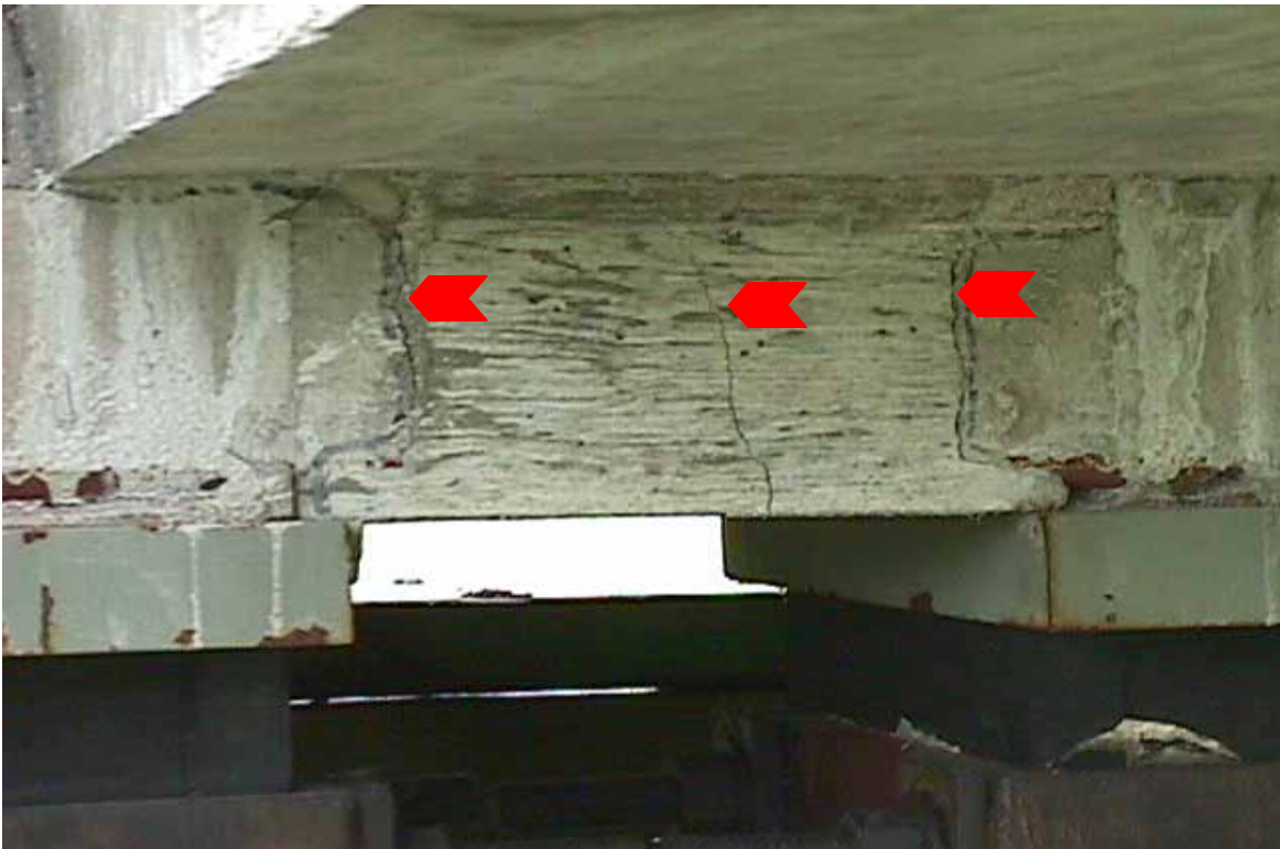
Figure 3-22. Cracking of diaphragm over center pier in concrete beam.
