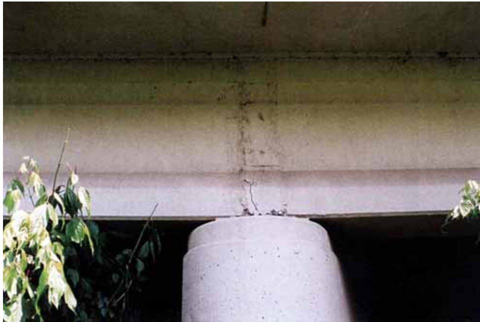
Figure 3-35. Bridge 2—cracking of diaphragm over pier.
