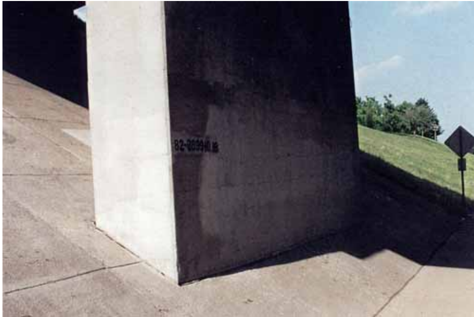
a. Flexural cracks visible on the pier.
