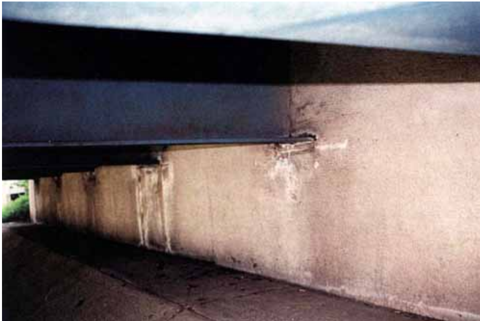
Figure 3-38. Bridge 7—efflorescence at construction joint.
