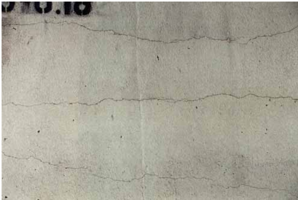
b. Closeup of flexural cracks on the pier.
