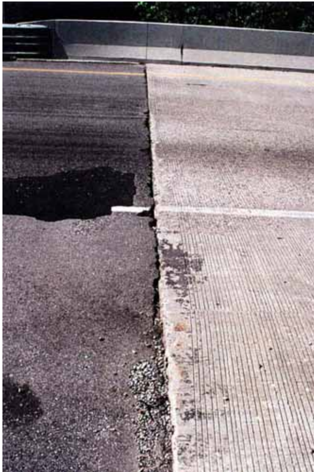
Figure 3-43. Bridge 5—interface of asphalt pavement and abutment wall without the use of an approach slab.
