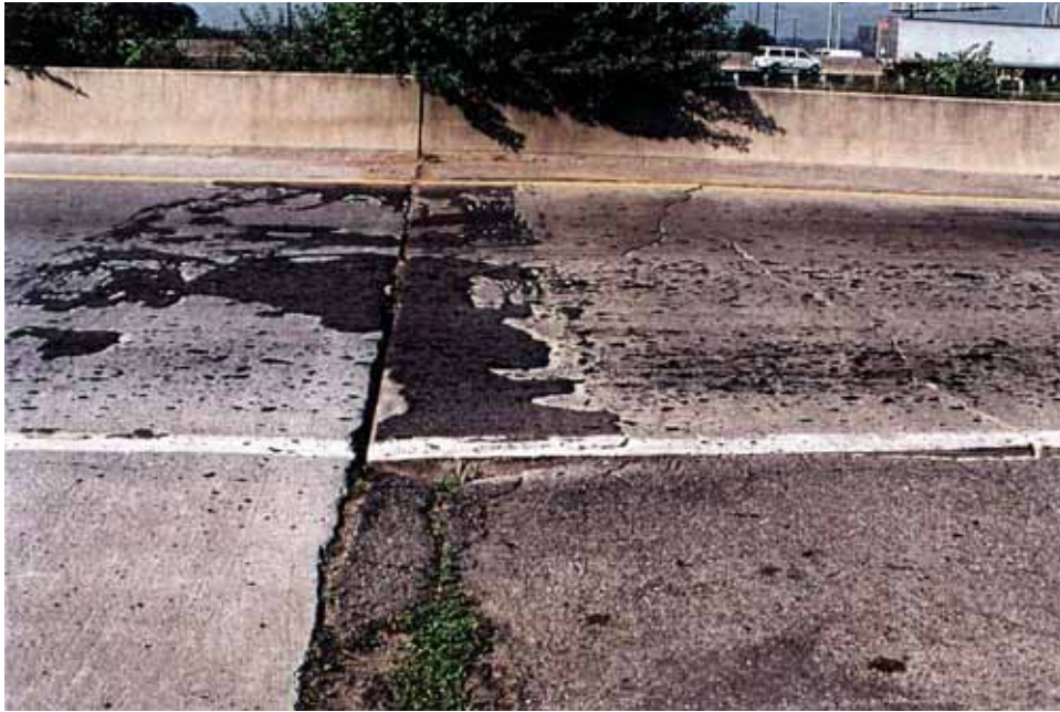
Figure 3-46. Bridge 7—patching at the end of approach slab.
