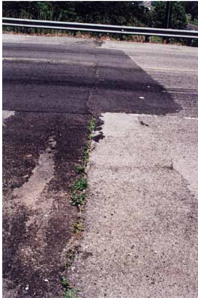
Figure 3-47. Bridge 10—patching at the end of approach slab (north side).
