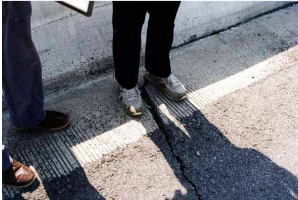
Figure 3-44. Bridge 1—opening between edge of approach slab and back face of abutment.
