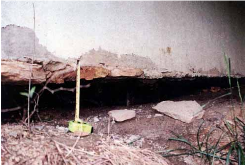
Figure 3-39. Bridge 6—washout under the abutment.
