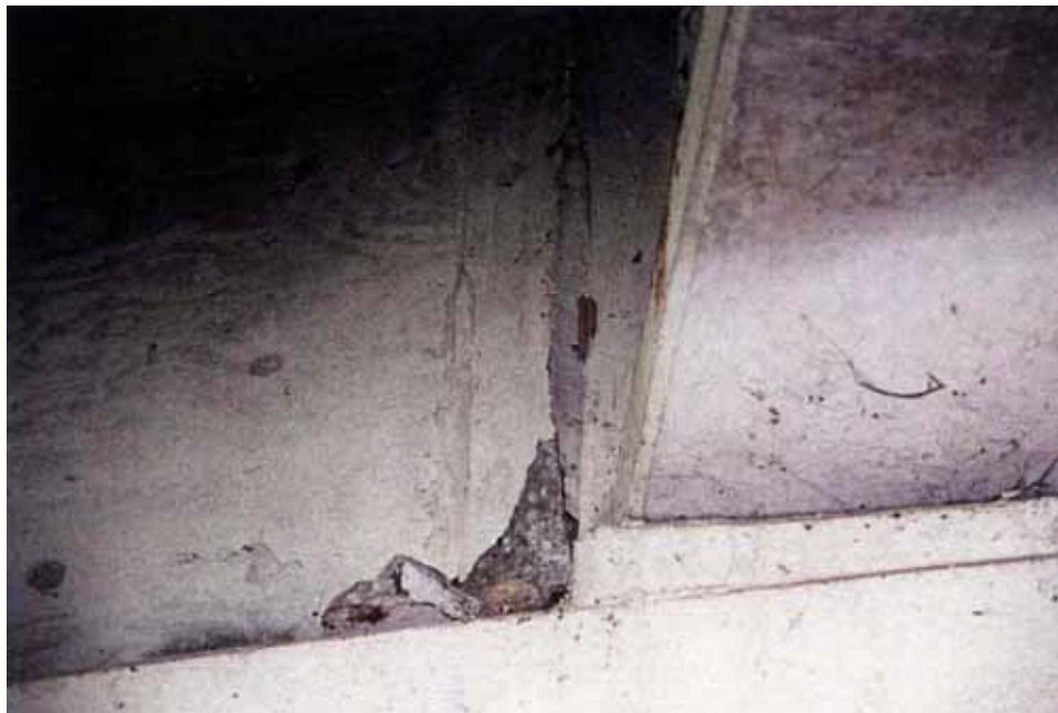
Figure 3-36. Bridge 2—cracking at interface of girder and pier diaphragm.
