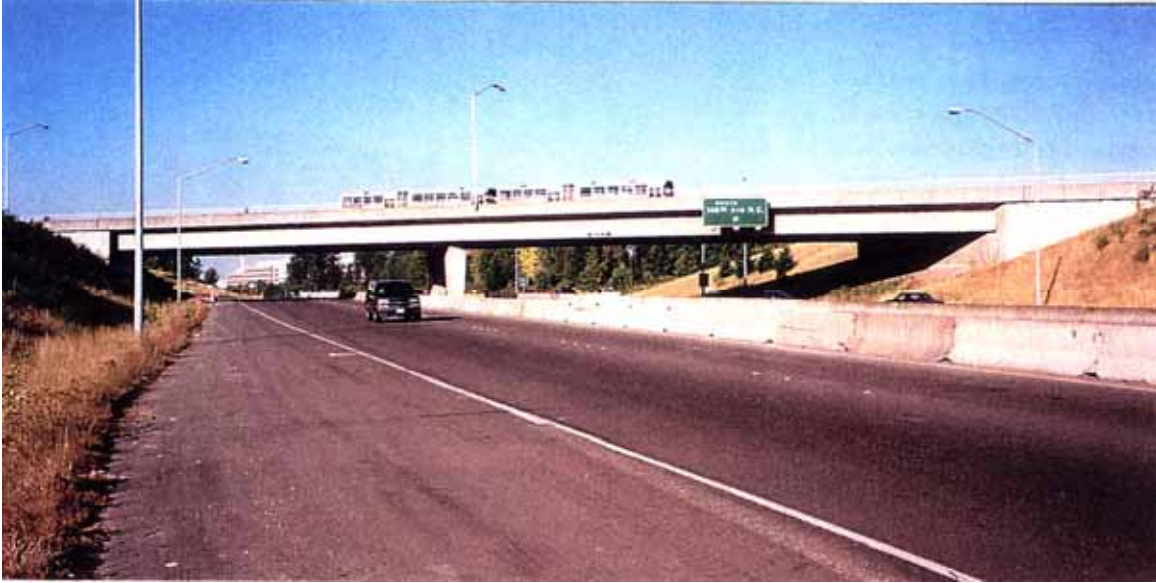
Figure 4-17. Two-span bridge with an overall length of 89 m (292 ft), a width of 11.6 m (38 ft), and a 45° skew. (52)
