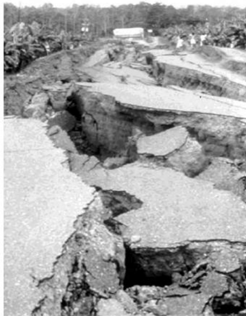
Figure 12-20 Disrupted fill and pavement due to liquefaction in Rio Estrella, Costa Rica during 1991 earthquake (Kavazanjian, et al., 2011).
