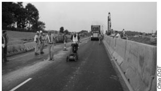
Figure 12-17 Use of GPR to check for voids beneath a pavement during work to repair a mine (Lefchik, et al., 2003).
