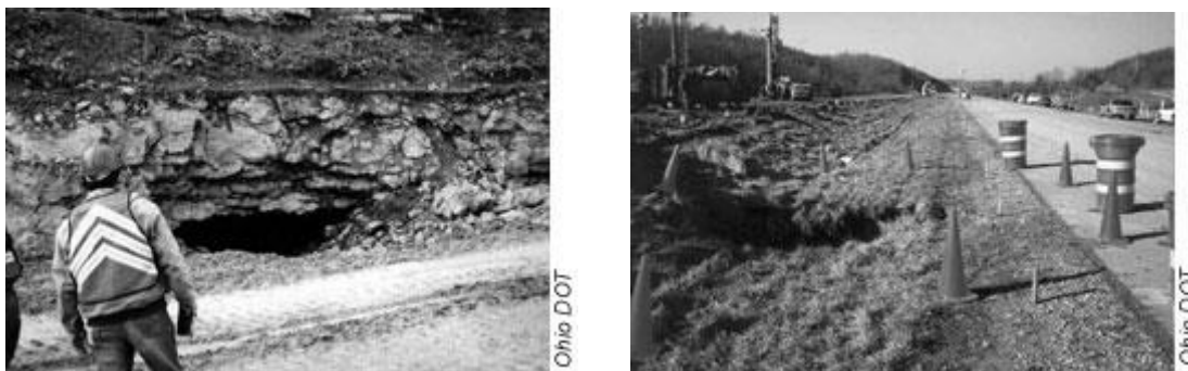
Figure 12-15 Surface effects from subsurface mines in Ohio: (a) I-470 and (b) I-70 (Lefchik, et al., 2003).
