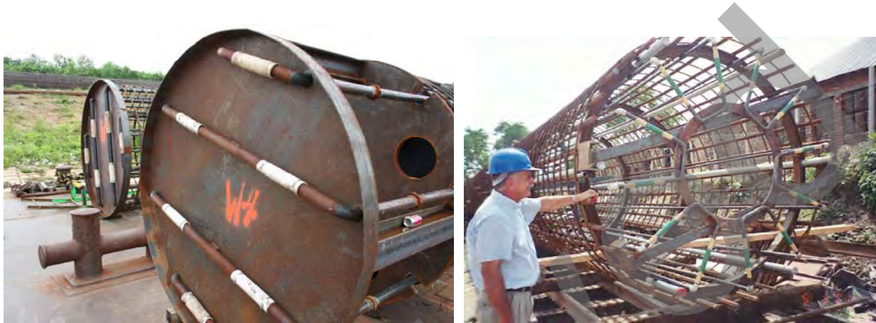
Figure 9-19 Sleeve Port Systems for Distribution of Grout to the Base of the Shaft
