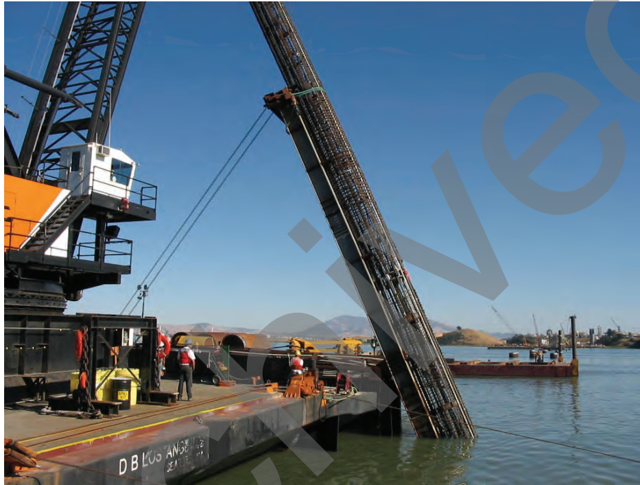
Figure 8-22 Photograph of Rebar Cage Being Lifted with a Tipping Frame (photo courtesy Malcolm Drilling)
