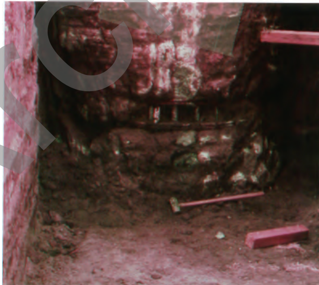
Figure 20-9 Defect Similar to the Defect that Produced the Logs in Figure 20-8 (Courtesy of Caltrans)
