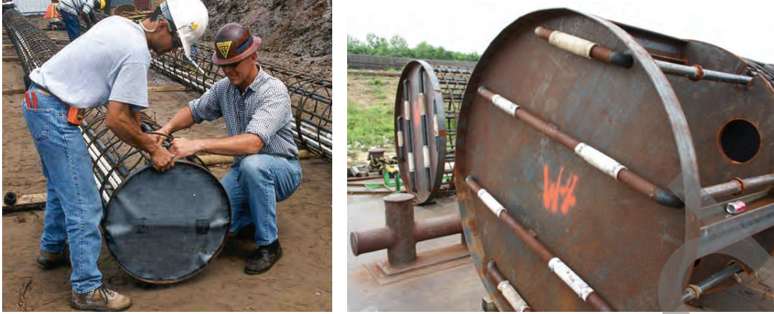
Figure 4-21 Base Grouting Systems Tied to Reinforcing Cage: Flat-jack method (left) and Tube-a-manchette method (right)
