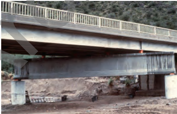
Figure 21-3 Use of Straddle Shafts to Replace an Existing Foundation (photo by B. Berkovitz)
