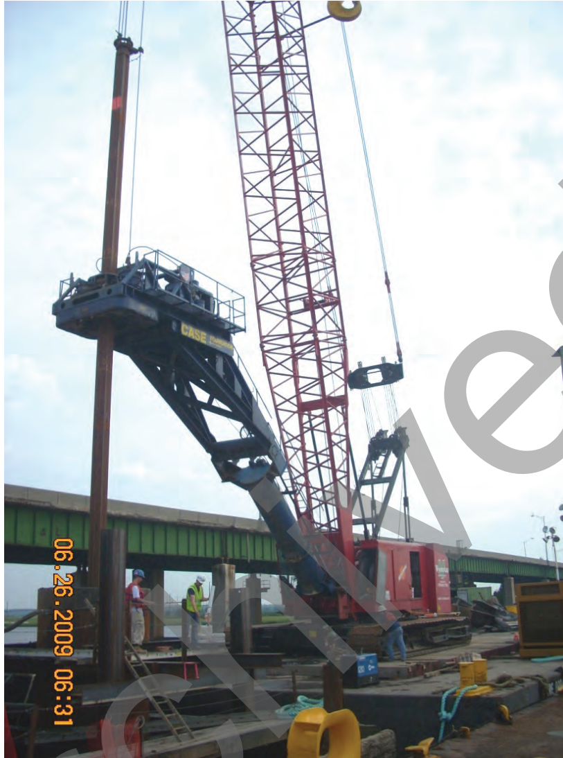
Figure A-12 Crane-Mounted Drilling Machine for Construction Over Water (Photo courtesy of Paul Axtell)
