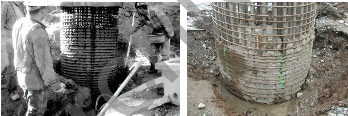
Figure 8-6 Examples of Inadequate Flow of Concrete through Tightly Spaced Spiral Reinforcement
