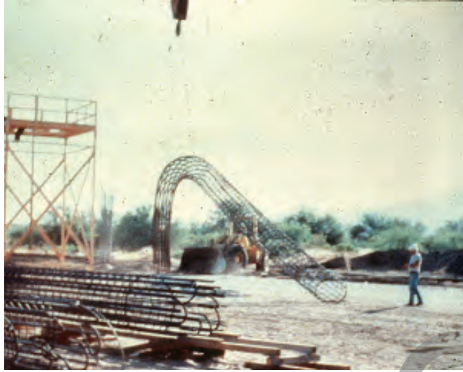
Figure 8-20 Photograph of Rebar Cage Being Lifted Improperly (Photo courtesy of Barry Berkovitz, FHWA)
