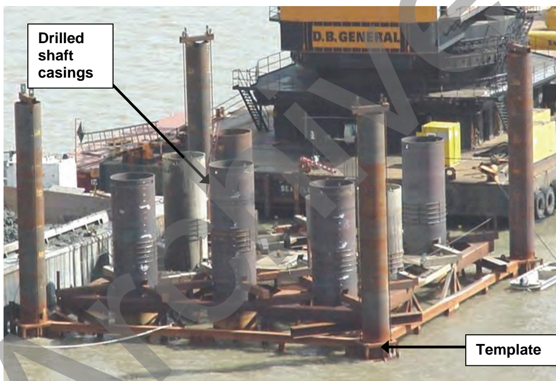
Figure 14-1 Group of Drilled Shafts During Construction of the Benetia-Martinez Bridge near San Francisco
