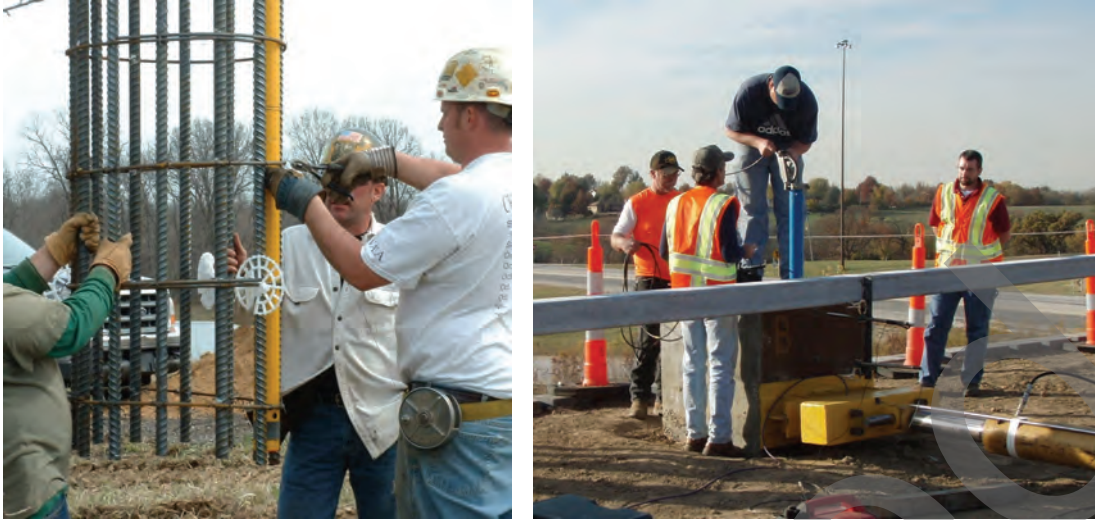
Figure 17-62 Measurements of Lateral Displacement in a Lateral Test Shaft below Grade Using an Inclinometer
