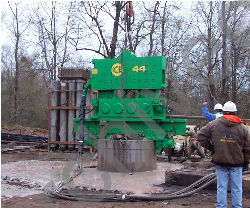
Figure 9-5 Slurry Displaced from Annular Space during Casing Extraction
