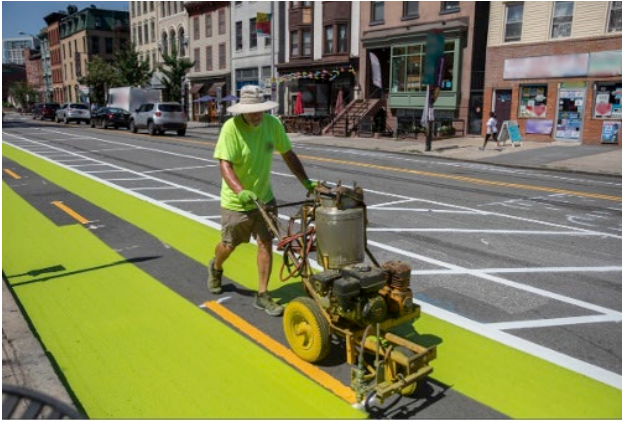
© 2024 Jersey City Department of Infrastructure. A. Striping of two-way separated bike lane.
