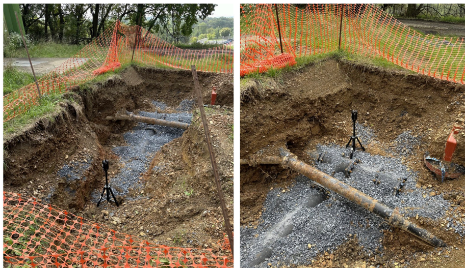
Figure 3. Photos. Example potential scan positions to cover inside a trench with a lightweight terrestrial lidar scanner.
