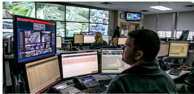
Figure 1. Photo. A traffic operations center in Chester, VA.
