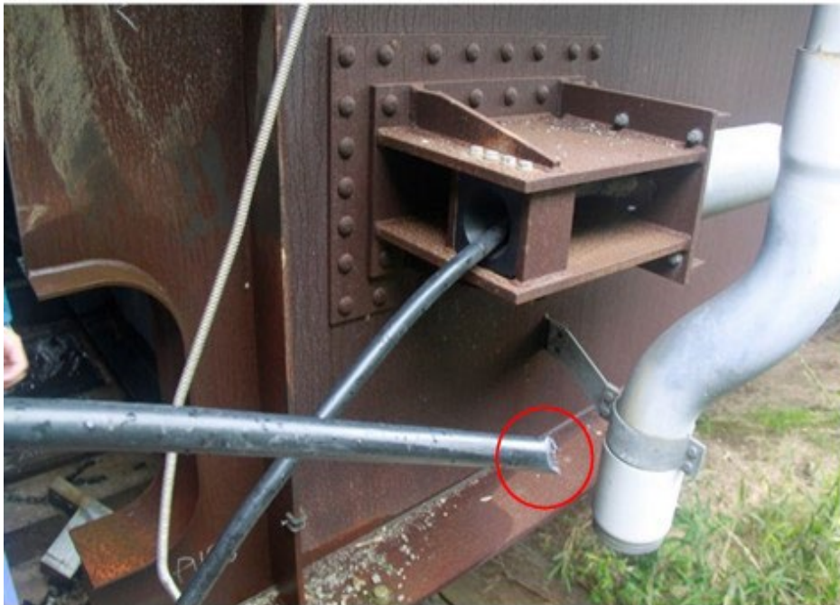
Figure 21. Photos. Bearing failure below each girder starting from the outside girder G1 to the inside girder G5 at abutment A1.
