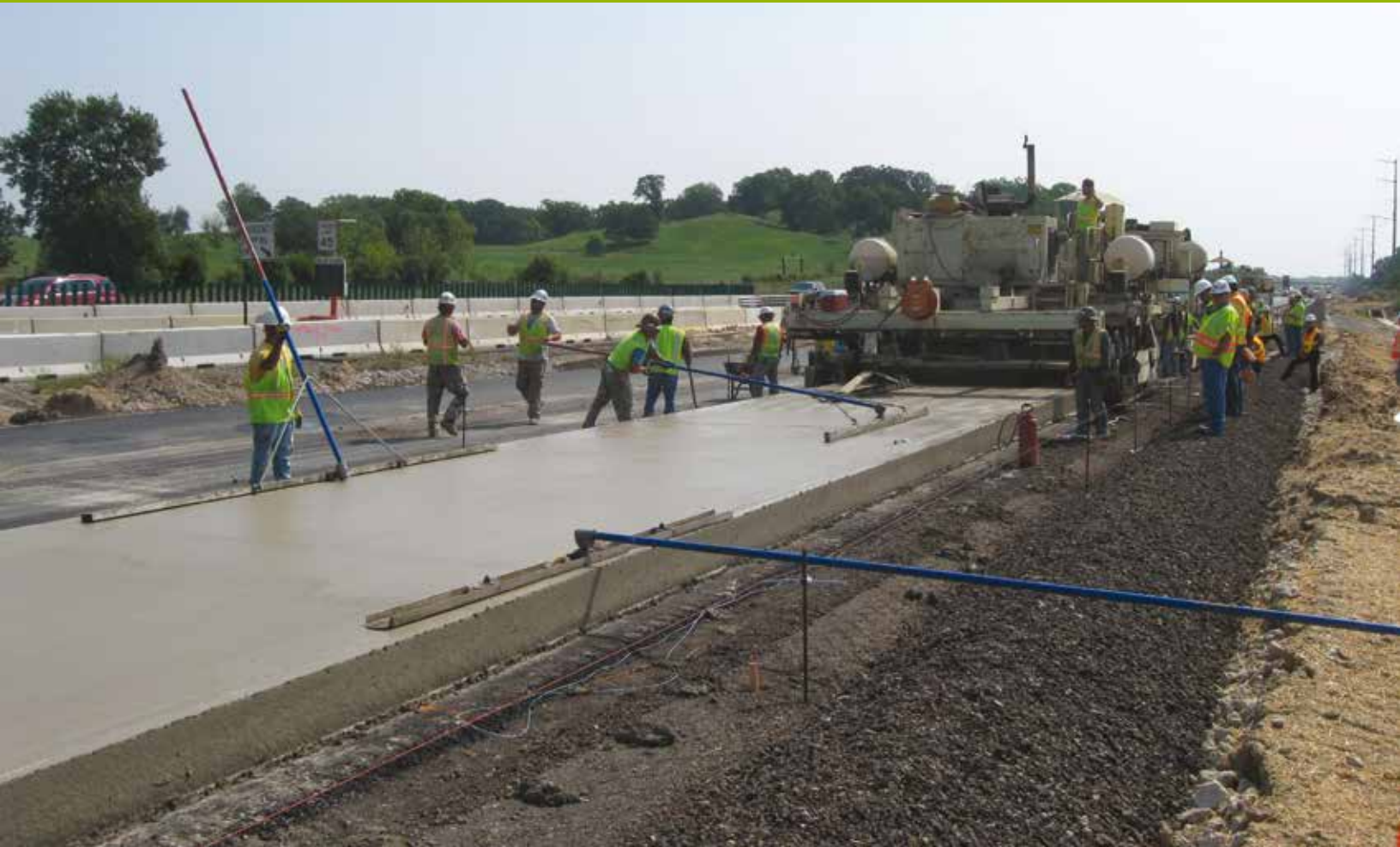
Figure 4. Photo: Workers place concrete with a slip form concrete paver. Source: FHWA.
