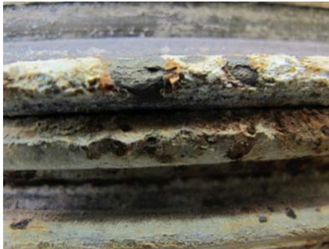
Figure 136. Photo. Close-up view of pit.
