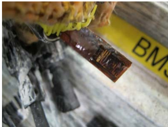
Figure 168. Photo. Corroded LPR sensor 5.
