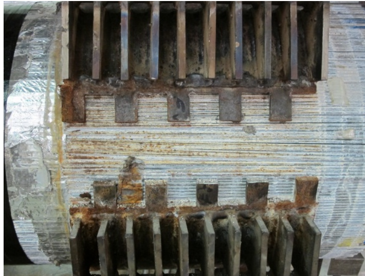
Figure 141. Photo. South end of cable highlighting teeth of cable band.
