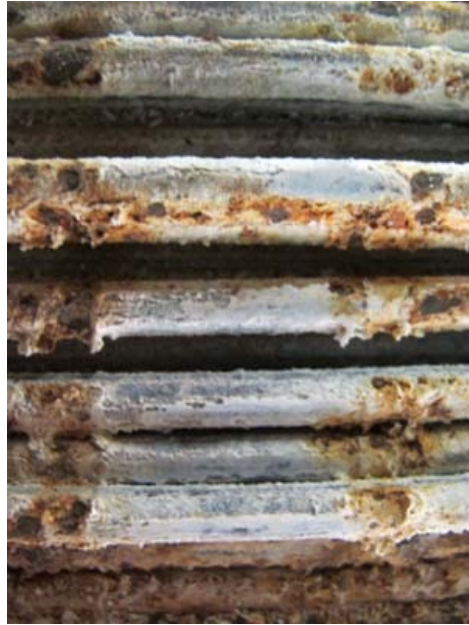
Figure 135. Photo. Pitting corrosion under stainless steel strap.
