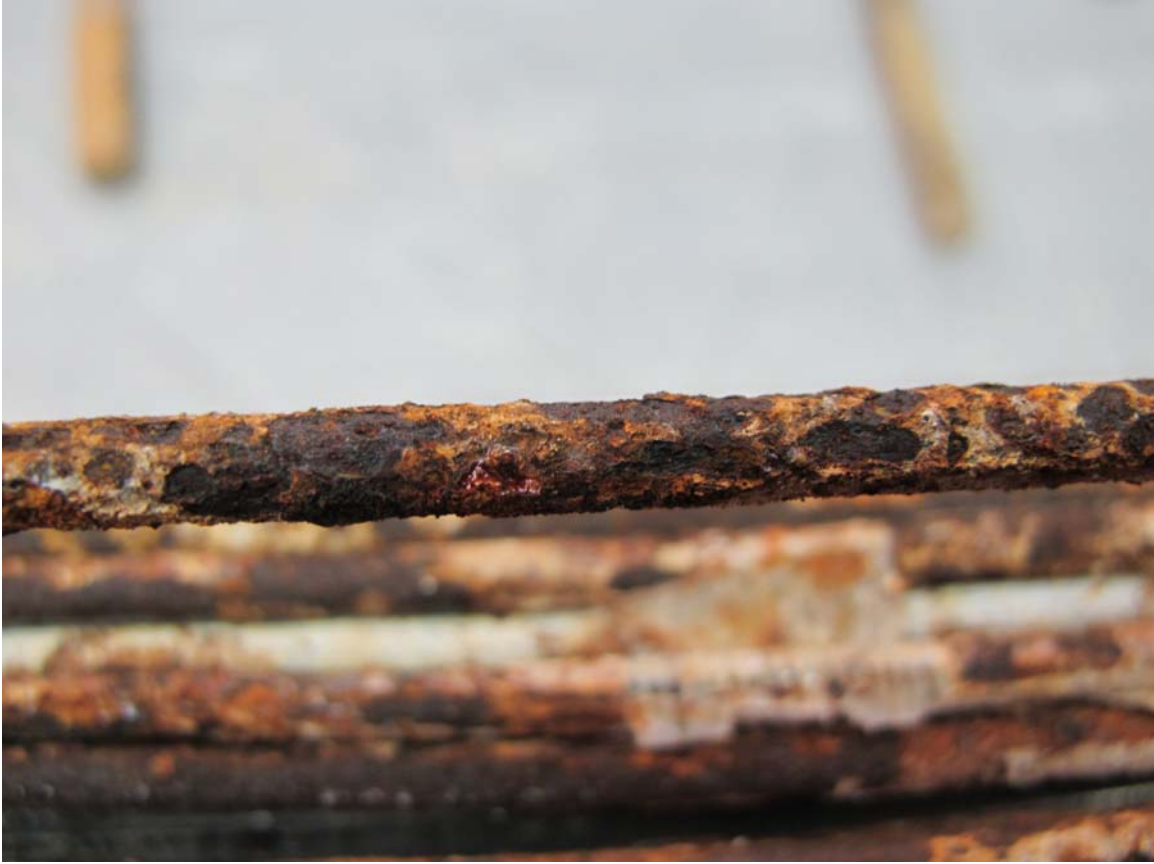
Figure 133. Photo. Close-up view of corroded wire.
