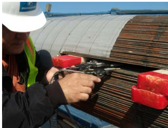
Figure 211. Photo. Decommissioning of the monitoring system by wedging the cable and pulling the sensors out.
