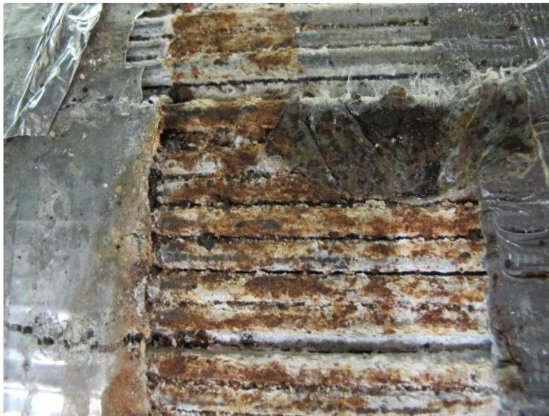
Figure 140. Photo. Wires at south end of cable with large percentage of stage 3 corrosion.
