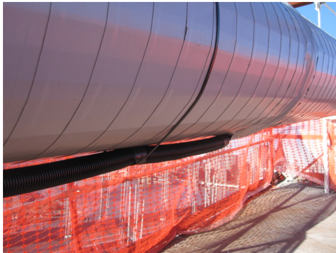
Figure 197. Photo. Cable temporary wrapping with neoprene and main conduit exiting at the bottom of cable leading to the main DAQ box at roadway level.
