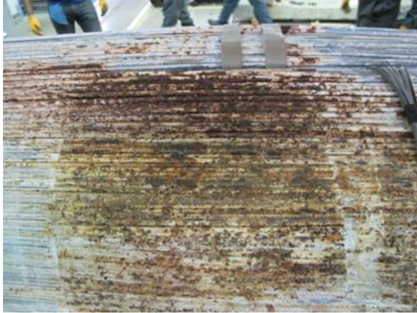
Figure 131. Photo. Close-up view of corroded area under neoprene wrapping.
