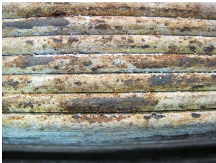
Figure 152. Photo. North end of cable close-up of 16R showing stage 3 corrosion.
