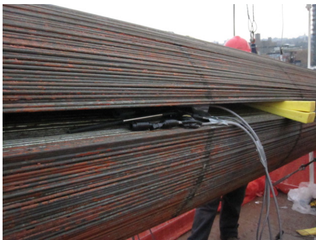
Figure 194. Photo. Sensor array used in each groove opening consisting of temperature/humidity sensors and LPR, CMAS, and BM corrosion sensors.
