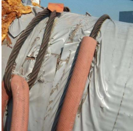
Figure 210. Photo. Damaged neoprene wrapping due to construction activity on the bridge.
