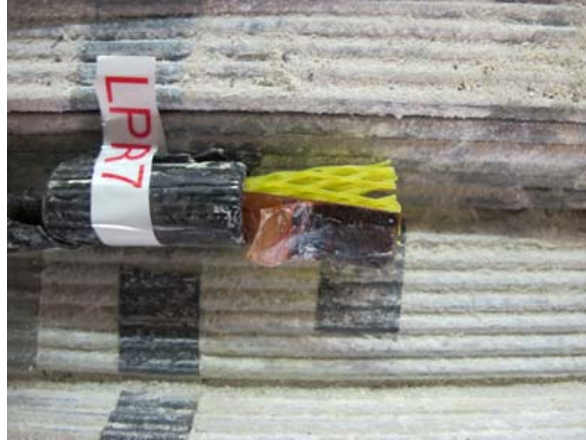
Figure 169. Photo. Corroded and disfigured LPR sensor 7.
