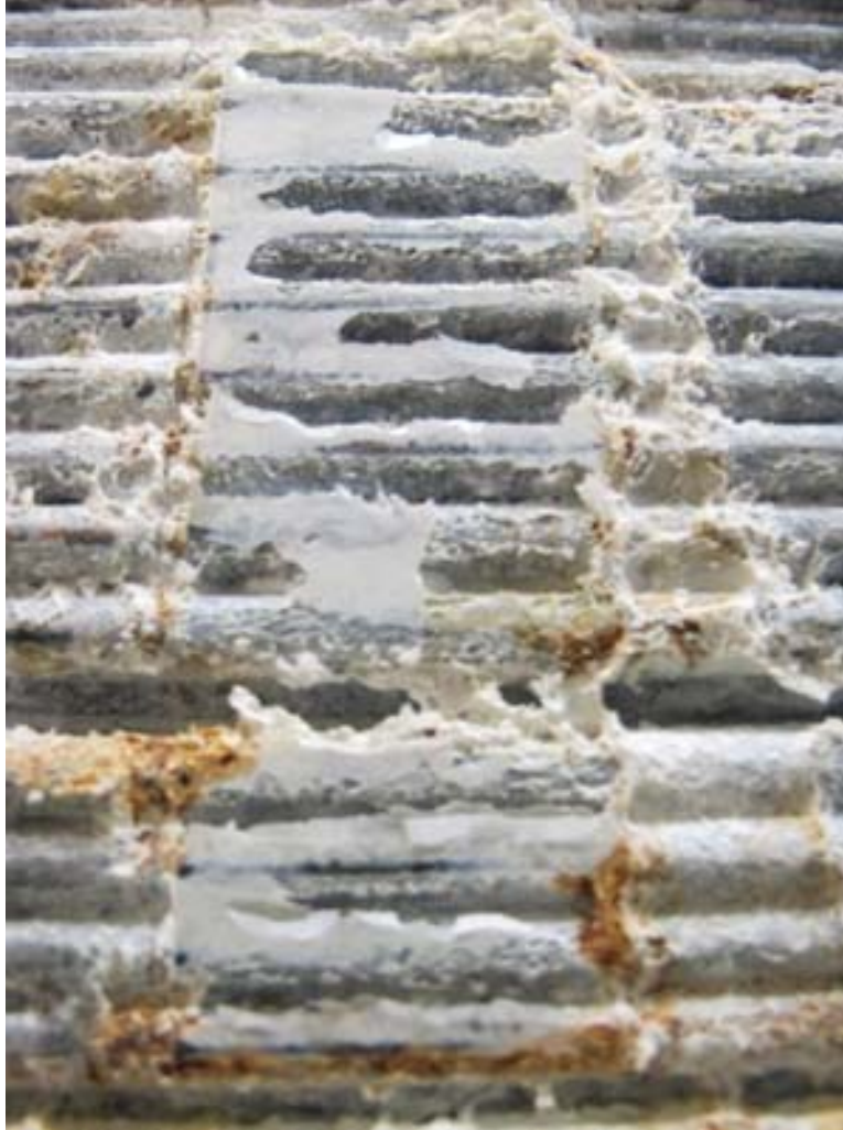
Figure 134. Photo. Salt build-up and zinc/ferrous corrosion product.
