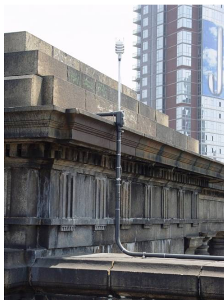
Figure 181. Photo. Weather station installed on the Manhattan Bridge.
