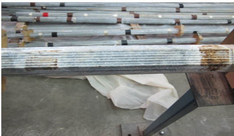
Figure 149. Photo. Corrosion formation at nylon strip location.
