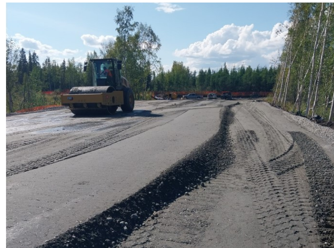
Below: Final lift of Select Borrow Type B on Northlake Lane extension at Cinch St.
