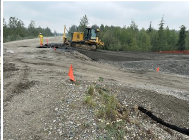
Below: Placing Select Borrow Type B on Northlake Lane extension at Cinch Street.
