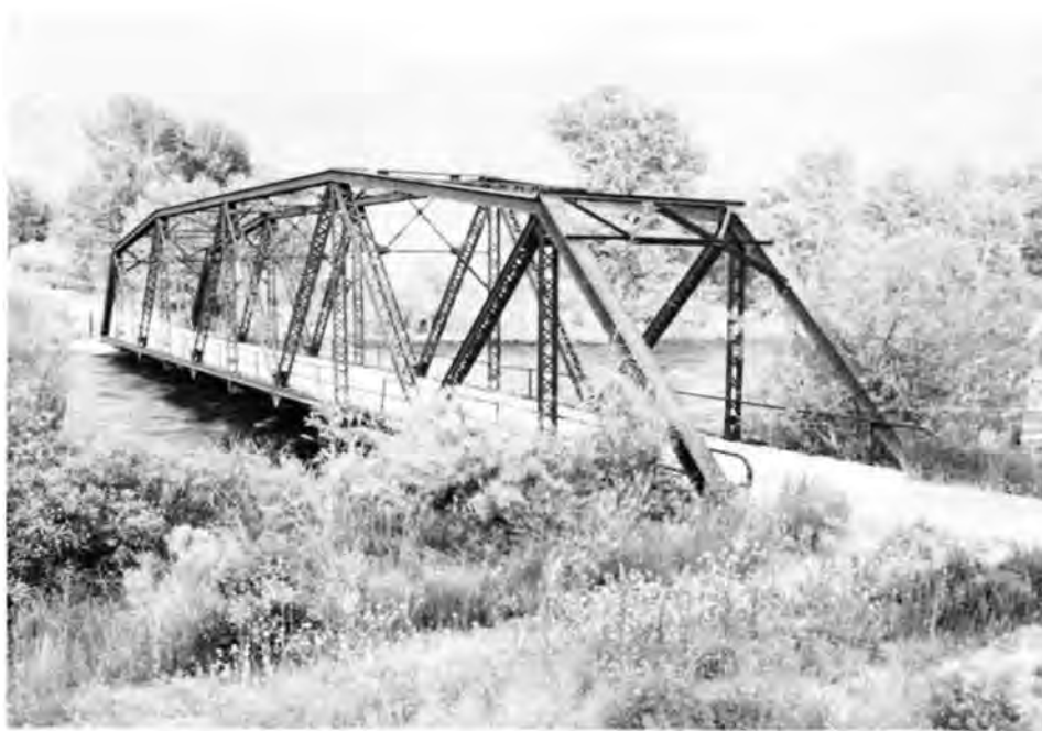
The present Browne's Bridge (Description 1) was built according to Montana State Highway Commission standardized plans. (Photograph Fred Quivik).
