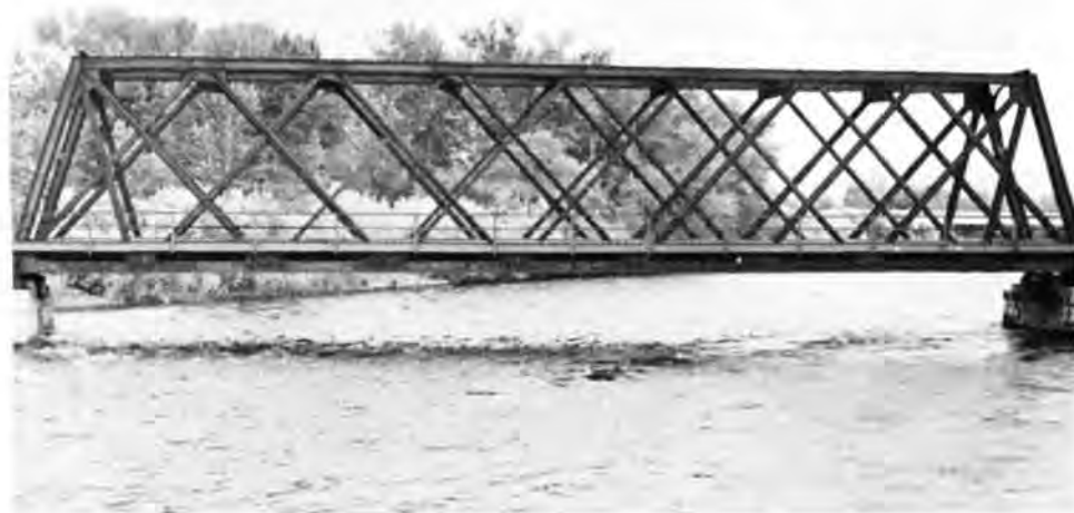
The Union Pacific bridge (Description 2) over the Big Hole River near Glen was built in 1901 by the American Bridge Company. It and two other Union Pacific bridges built elsewhere in Beaverhead County in 1902 are the only triple intersection Warren trusses in Montana. (Photograph Fred Quivik).
