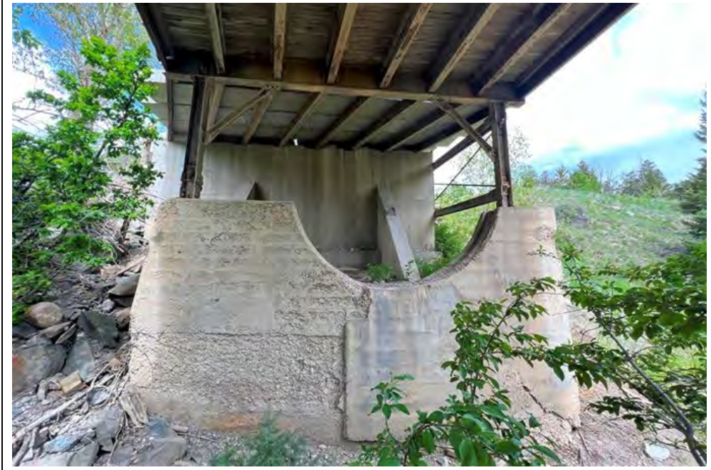
Figure 9. Sun River Bridge (24TT199), underside of deck at west abutment, pipe saddle; view southwest. Photo by Jeannie Larmon, 5/24/2023.
