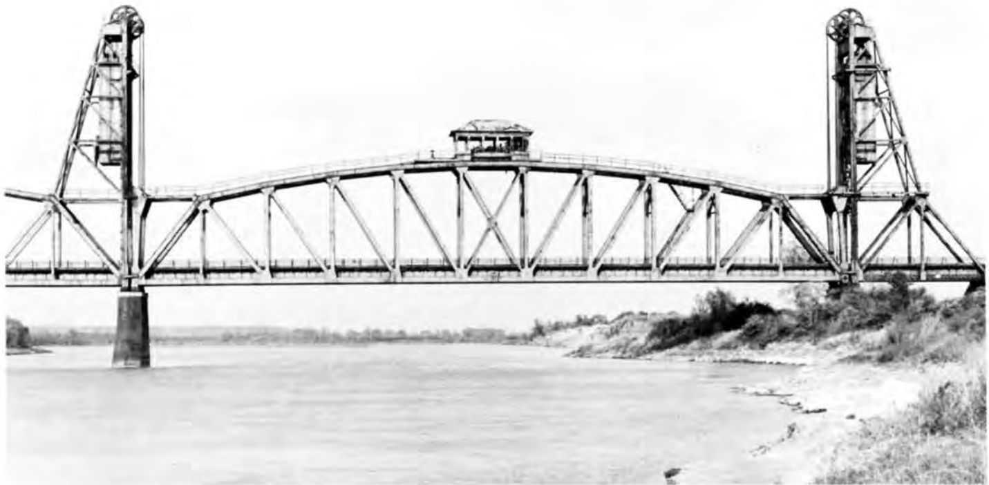
The 296-foot lift span of the Snowden Bridge (Description 65) was necessitated because the Missouri River was still considered a navigable river at this point in 1913. Designed by Waddell and Harrington of Kansas City, the bridge was the longest lift span in the world at the time of its construction. (Photograph Jet Lowe).
