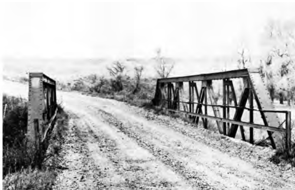
The Judith River Bridge (Description 21) is a riveted Warren pony truss, the most commonly used structural type of those covered by the Montana Historic Bridge Inventory. (Photograph Jet Lowe).
