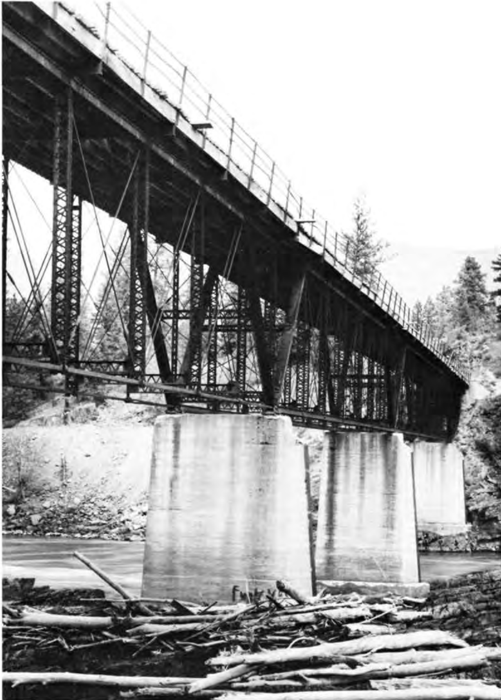
The Main Channel Bridge (Description 67) was built in 1911 in association with the Thompson Falls Power Plant downstream. (Photograph Jet Lowe).
