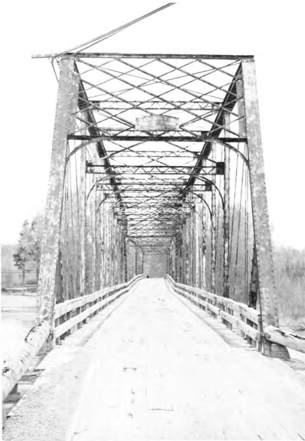
The Old Steel Bridge (Description 23) over the Flathead River at Kalispel is a three-span, pin-connected Pratt through truss bridge built by Gillette-Herzog of Minneapolis in 1894. It is the oldest surviving bridge in northwestern Montana. (Photograph Jet Lowe).
