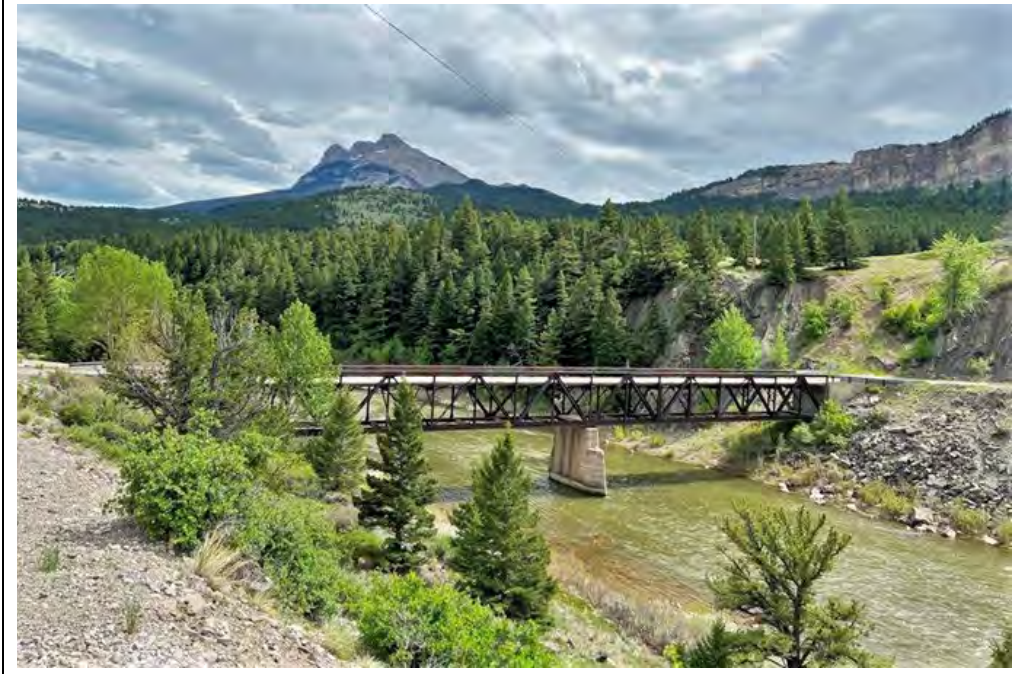
Figure 5. Sun River Bridge (24TT199), northwest face; view south. Photo by Jeannie Larmon, 5/24/2023.
