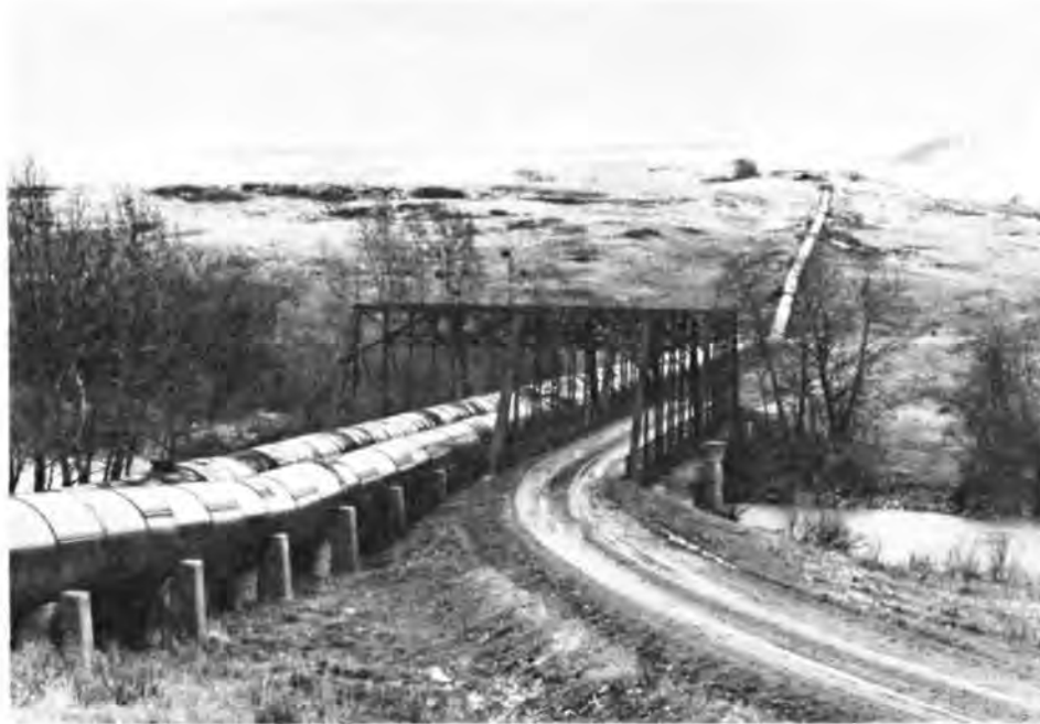
The St. Mary River Bridge (Description 30) carries water from the St. Mary River to the Milk River as part of an early 20th Century irrigation project. (Photograph Jet Lowe).
