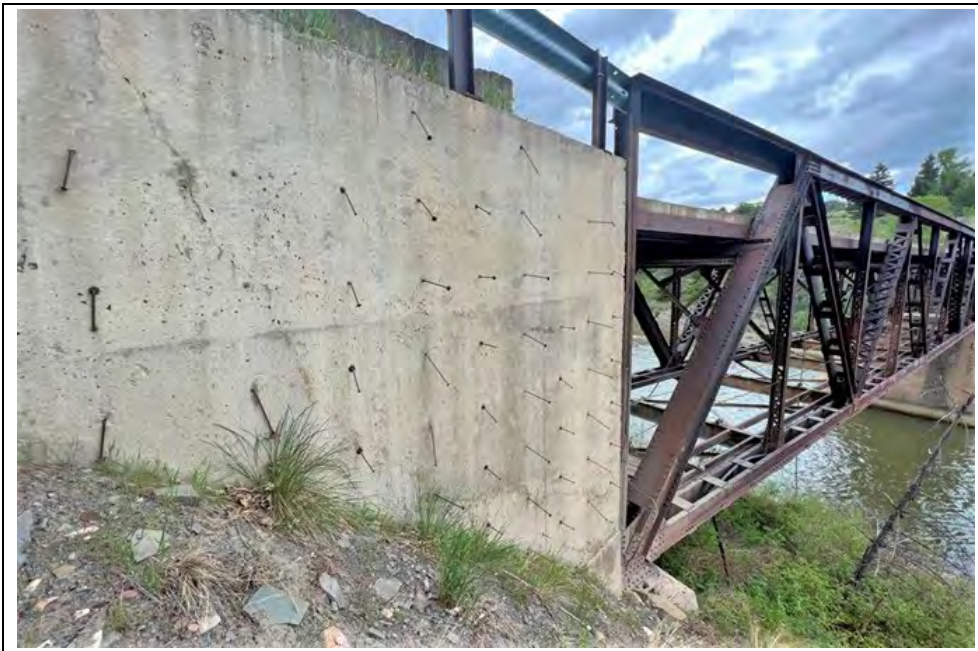
Figure 8. . Sun River Bridge (24TT199), detail of west abutment, south face; view northwest. Photo by Jeannie Larmon, 5/25/2023.
