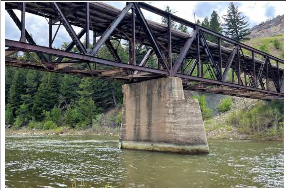
Figure 7. Sun River Bridge (24TT199), northeast face of central pier; view southwest. Photo by Jeannie Larmon, 5/24/2023.
