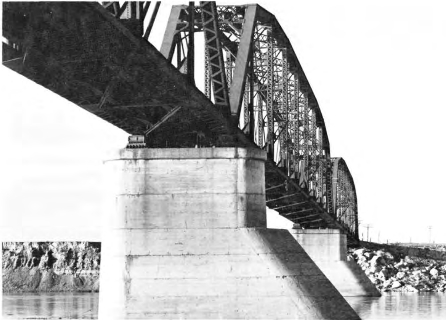
The use of reinforced concrete in bridge piers, approach spans, and smaller bridges was a major contribution of the Milwaukee Road to Montana bridge building. These massive piers support the Calipso Bridge (Description 60). (Photograph Jet Lowe).
