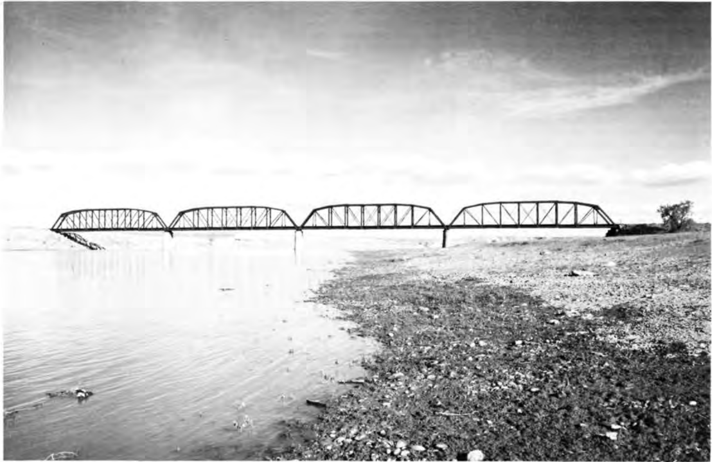
Calipso Bridge (Description 60) over the Yellowstone River west of Terry. (Photograph Jet Lowe).
