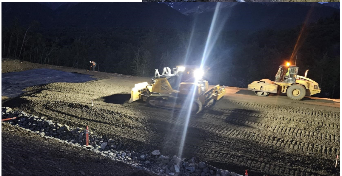
Bottom: Compacting select borrow for traffic at the end of a shift.
