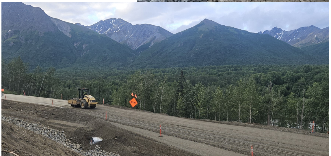
Bottom: Compacting select borrow for traffic at the end of a shift.
