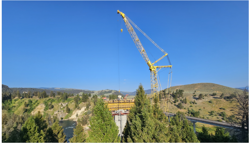
Daytime picture of concrete pour with Yellowstone River, the new construction and the old bridge
