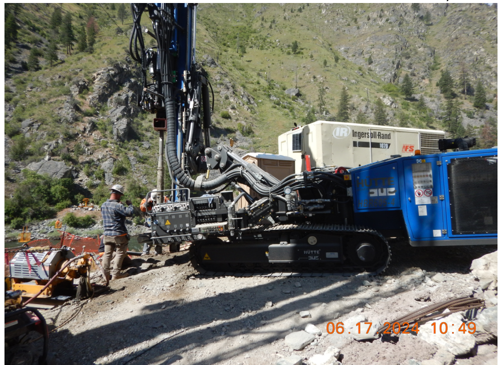
Preparing Drill rig for installation of PGA casings at EAB Source of photos: FHWA
