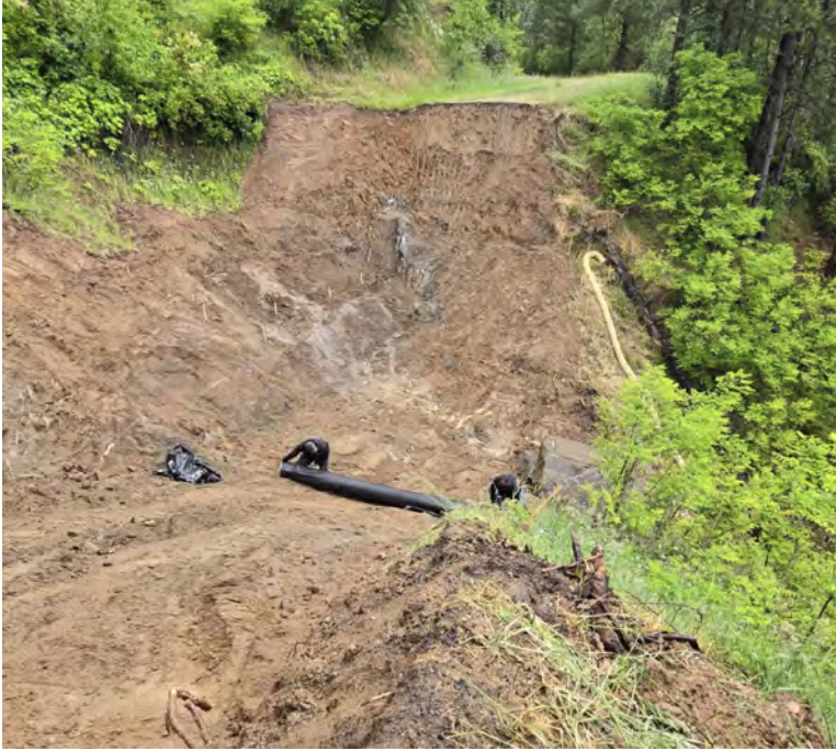
Slide excavation, FSR 5503 M.P. 1.28
