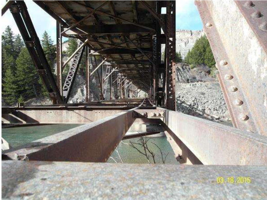
PHOTO #7 MTA-SR-001, SUN RIVER BRIDGE, PHOTO BY GARY GRASSEL. THIS PHOTO IS A VIEW LOOKING FROM THE LEFT ABUTMENT TO THE CENTER PIER ON THE UPSTREAM SIDE OF THE BRIDGE. NOTE THE SAG IN THE TRUSS APPROXIMATELY AT MID-SPAN OF THE UPSTREAM SIDE ONLY. CONNECTIONS HAVE BEEN INSPECTED BY RECLAMATION CLIMB TEAM AND NOTHING OUT OF THE NORMAL WAS OBSERVED AT THE CONNECTIONS OR MEMBERS. (03/18/2015)
