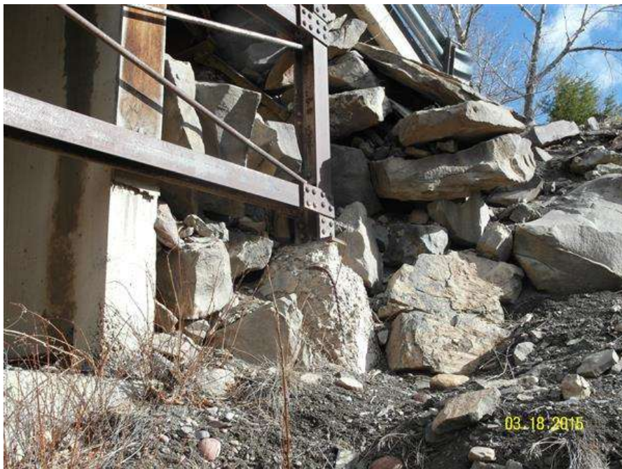
PHOTO #8 MTA-SR-001, SUN RIVER BRIDGE, PHOTO BY GARY GRASSEL. THIS IS A VIEW OF THE SUPPORT PIER ON THE LEFT DOWNSTREAM APPROACH SPAN OF THE BRIDGE. RECOMMEND REPLACING THIS EXISTING PIER WITH NEW REINFORCED CONCRETE PIER. (03/18/2015)
