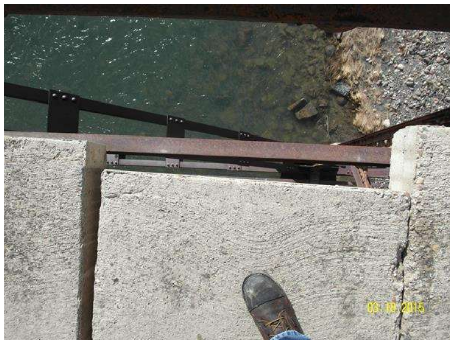
PHOTO #3 MTA-SR-001, SUN RIVER BRIDGE, PHOTO BY GARY GRASSEL. THIS PHOTO SHOWS THAT THE PRECAST FLOOR PLANKS ARE NOT FASTENED TO THE SUPERSTRUCTURE BEAM MEMBERS. PLANKS CAN MOVE UPSTREAM OR DOWNSTREAM AND MAY SHIFT A DISTANCE WHERE THEIR USE AS A TRAFFIC SURFACE WILL BE A CRITICAL FAILURE MODE. (03/18/2015)
