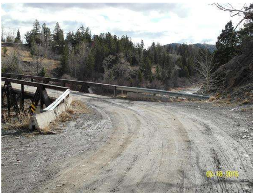
PHOTO #6 MTA-SR-001, SUN RIVER BRIDGE, PHOTO BY GARY GRASSEL. THIS IS A VIEW OF THE RIGHT APPROACH TO THE BRIDGE. (03/18/2015)
