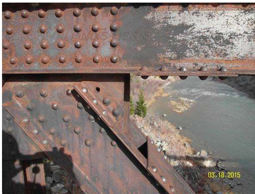
PHOTO #2 MTA-SR-001, SUN RIVER BRIDGE, PHOTO BY GARY GRASSEL. VIEW OF A MISSING FASTENER AT THE UPSTREAM SIDE, RIGHT TRUSS, FIRST TOP JOINT FROM THE RIGHT BEARING. (03/18/2015)
