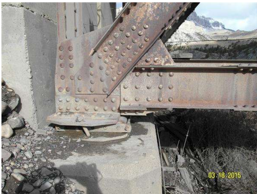
PHOTO #12 MTA-SR-001, SUN RIVER BRIDGE, PHOTO BY GARY GRASSEL. THIS IS A VIEW OF THE BEARING ASSEMBLY ON THE DOWNSTREAM SIDE OF THE RIGHT TRUSS AND RIGHT APPROACH. NOTE TRUSS ANCHOR BOLT IS BENT AND TRUSS BEARING PLATE COMING OFF THE ROLLERS. (03/18/2015)
