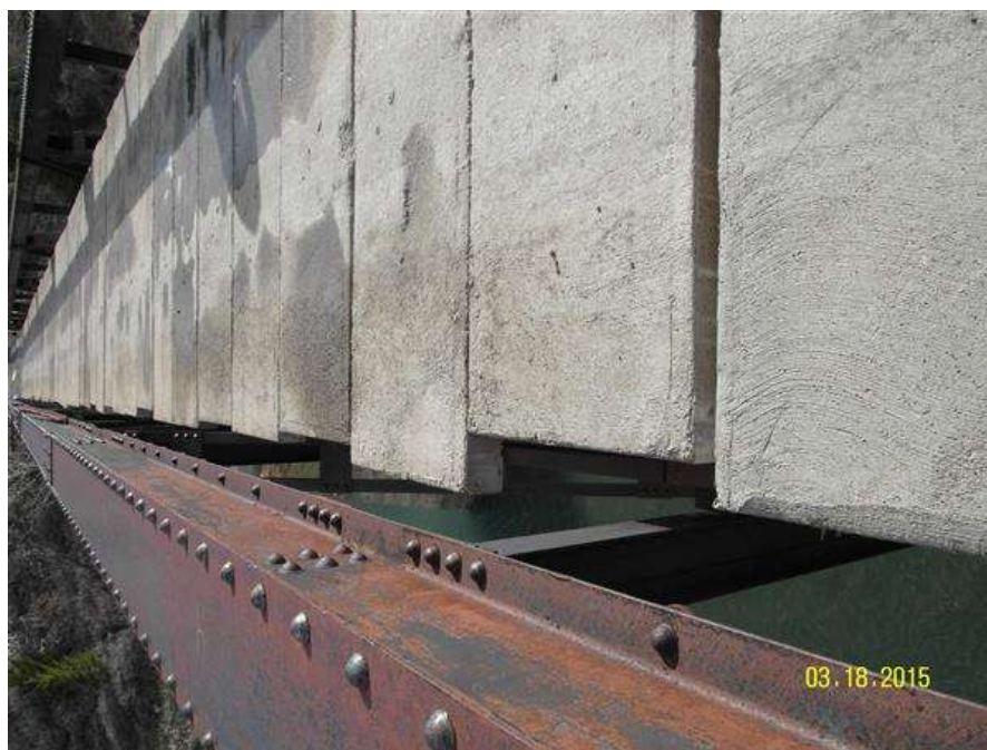
PHOTO #4 MTA-SR-001, SUN RIVER BRIDGE, PHOTO BY GARY GRASSEL. THIS PHOTO IS A VIEW PARALLEL TO BRIDGE CENTER LINE LOOKING AT THE DOWNSTREAM SIDE OF THE BRIDGE SURFACE. THE PRECAST PLANKS HAVE SHIFTED UPSTREAM AND DOWNSTREAM. RECOMMEND ALL PANELS ARE ATTACHED TO BEAMS AND ADJACENT PANELS TO CREATE NECESSARY DIAPHRAGM. (03/18/2015)
