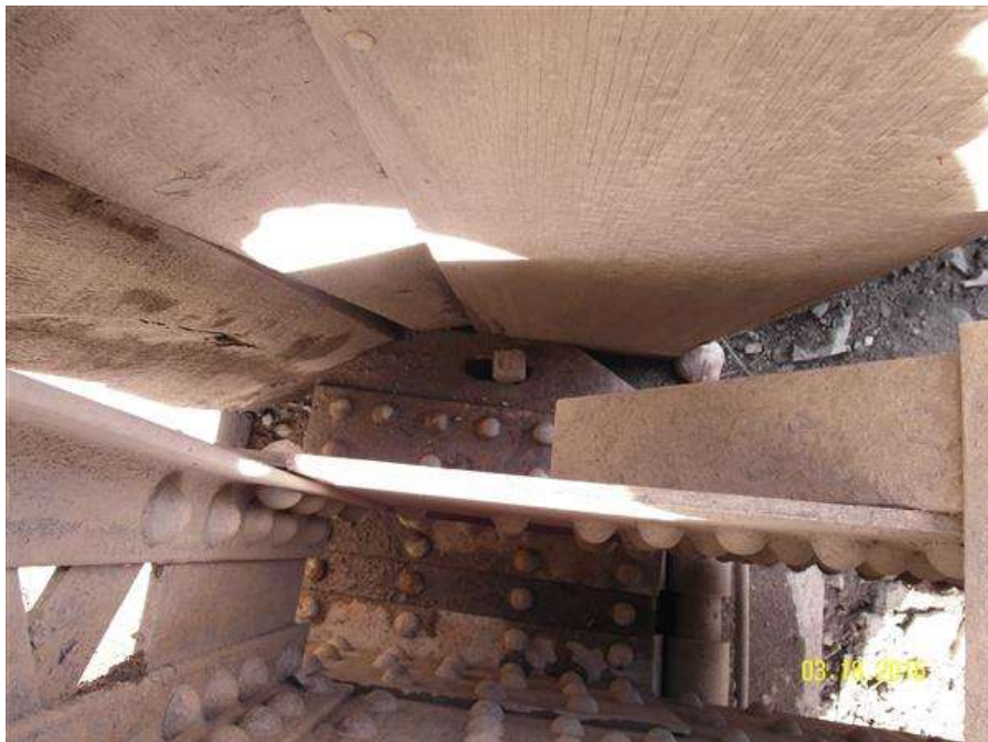
PHOTO #13 MTA-SR-001, SUN RIVER BRIDGE, PHOTO BY GARY GRASSEL. THIS IS A VIEW OF THE UPSTREAM SIDE AT THE SAME APPROACH AS IN PHOTO #12. THE ANCHOR BOLT IS BENT AND THE BEARING PLATE HAS EXTENDED PAST THE FIRST ROLLER. (03/18/2015)
