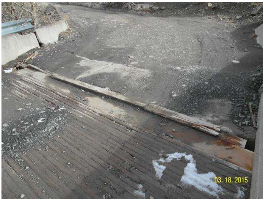
PHOTO #5 MTA-SR-001, SUN RIVER BRIDGE, PHOTO BY GARY GRASSEL. THIS PHOTO SHOWS THE LEFT (EAST) APPROACH SPAN OF THE BRIDGE. REPAIRS HAVE BEEN MADE SINCE THE LAST INSPECTION. (03/18/2015)
