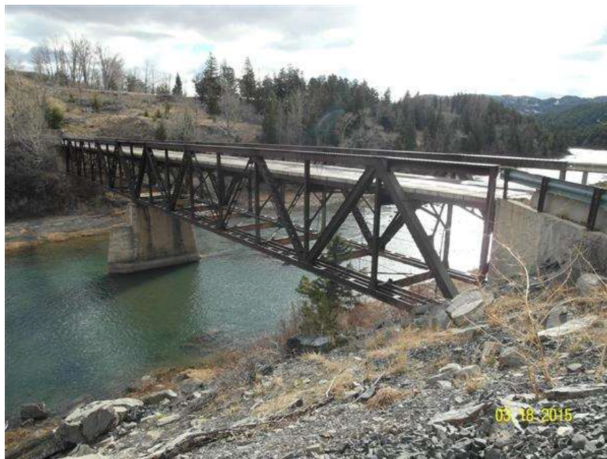
PHOTO #1 MTA-SR-001, SUN RIVER BRIDGE, PHOTO BY GARY GRASSEL. VIEW LOOKING AT THE UPSTREAM SIDE OF THE BRIDGE. (03/18/2015)
