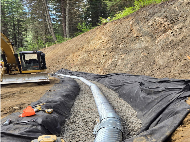
12-inch collector pipe M.P. 13.6 FSR354
