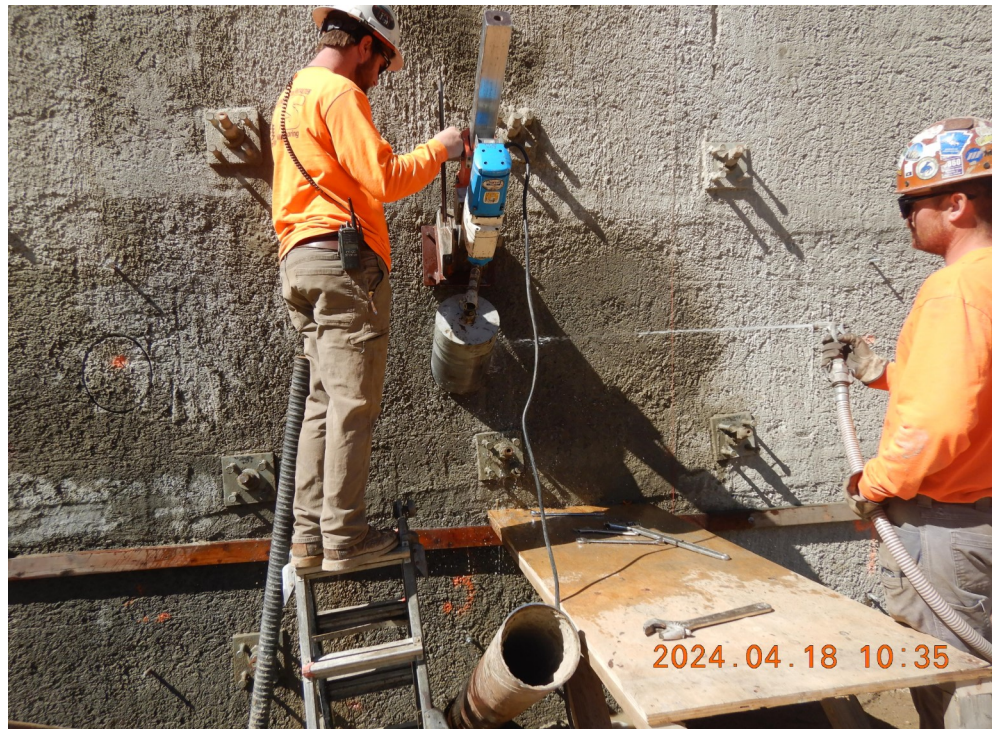
Core drilling through Soil Nail Wall for the Permanent Ground Anchors at abutment 1
