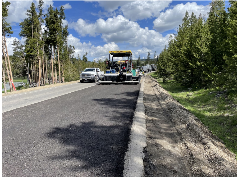
Above: The cold-in place pavement being placed behind the paver after it has gone through the mill and has had the emulsion mixed into the material.
