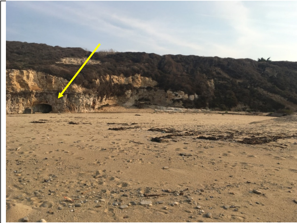
Bonny Doon Beach, culvert opening at the base of the cliff in left hand portion of photograph
