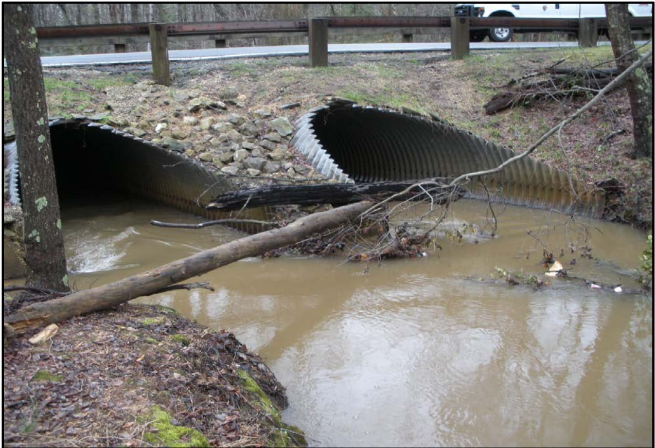
Figure 1. Corroded double culverts at Still Creek (upstream)
