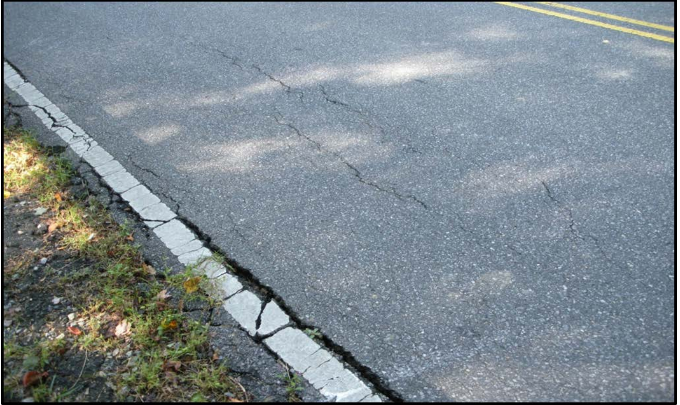
Figure 9. Roadway cracking and settling
