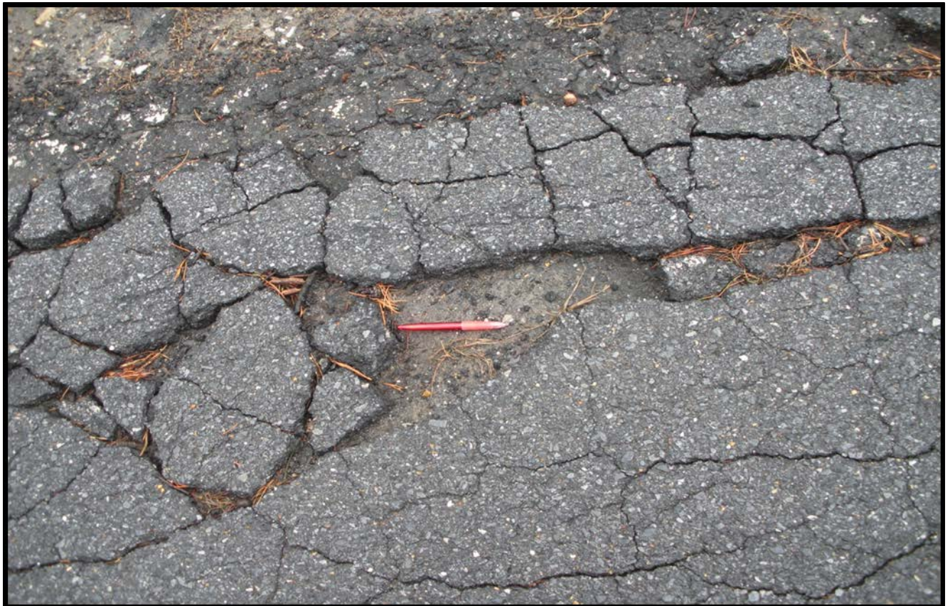
Figure 10. Edge of pavement cracking
