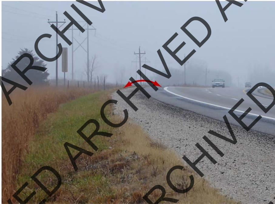
FIGURE 23 Cross-slope break on the high side of superelevated curve.
