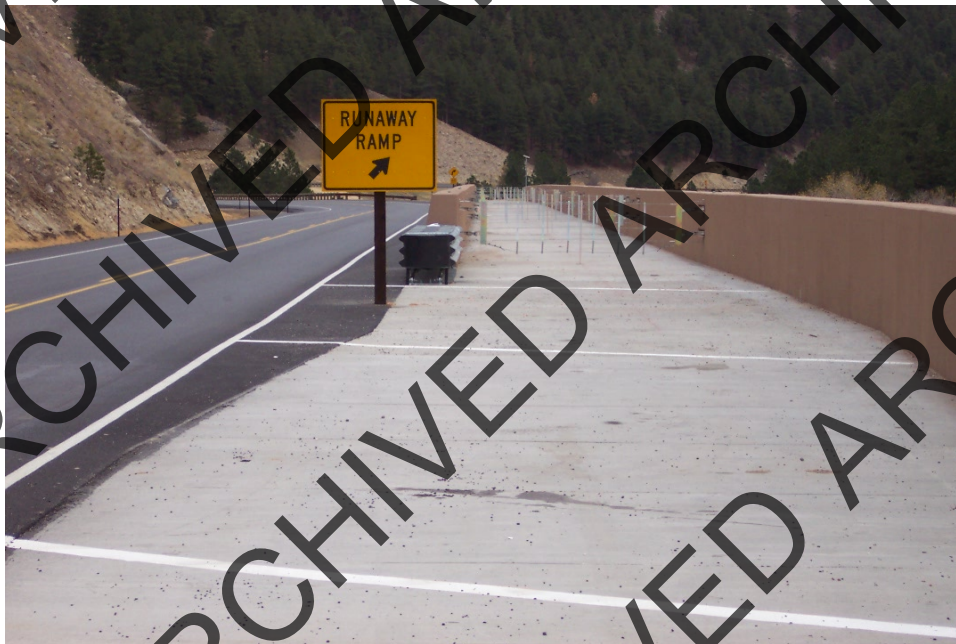
FIGURE 91 Runaway truck ramp with arrestor system.
