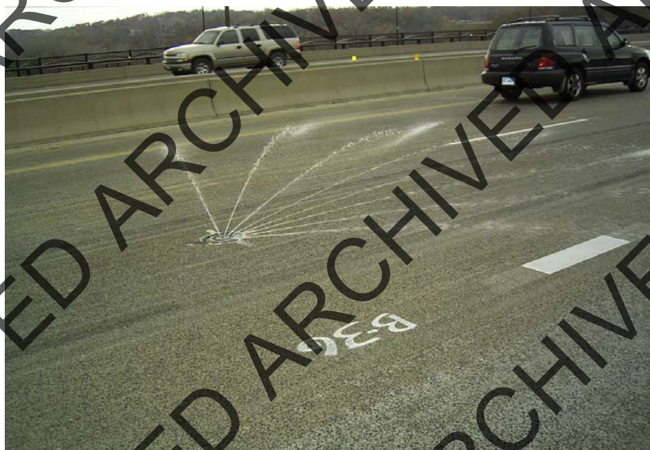
FIGURE 45 Anti-icing system on a bridge
