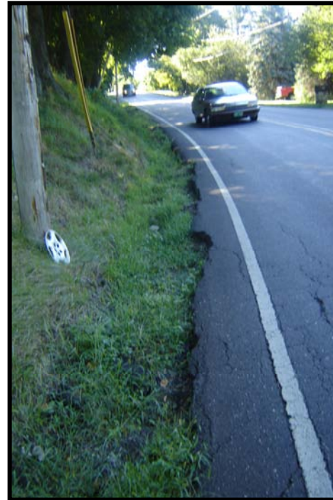
Drop off on the inside of curve – PA 412 at Slifer Valley Road
