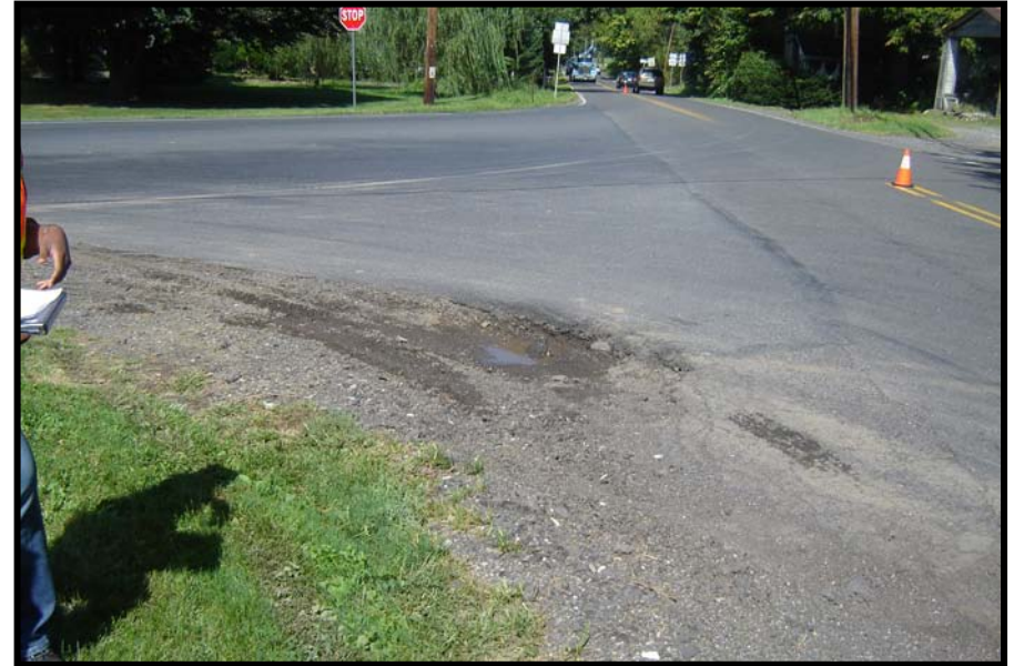
PA 412/PA 212 west intersection – standing water; poor turning radius
