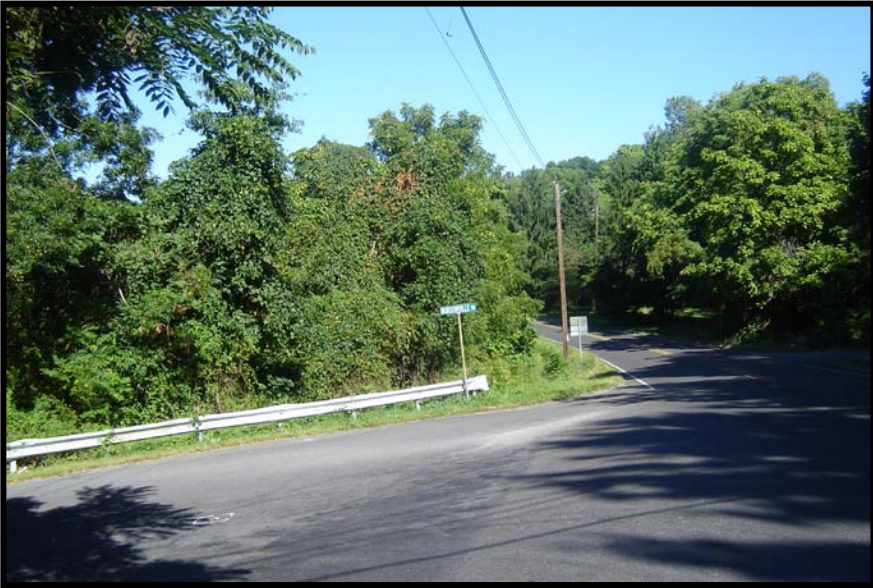
Sight distance at Bursonville Road is severely compromised. Curve north of Buckwampum Road is not delineated.
