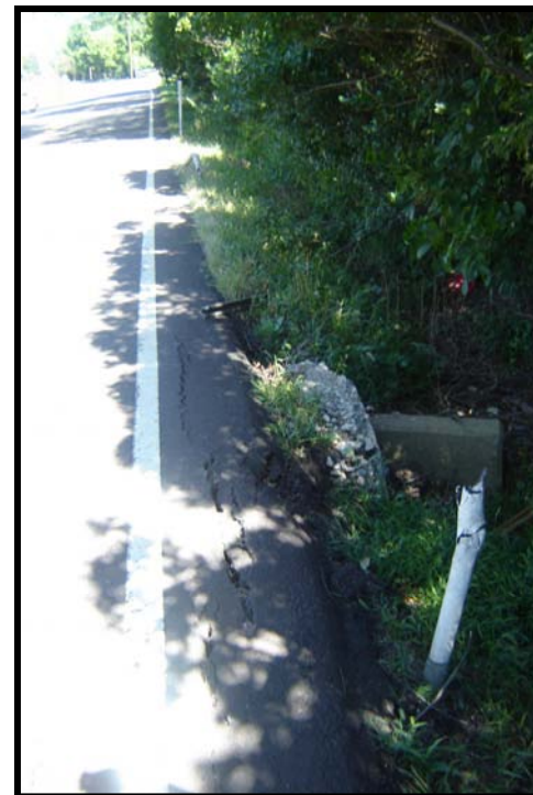
Drop off in the area between Park Drive West and Park Drive East. Delineator pole are damaged.
