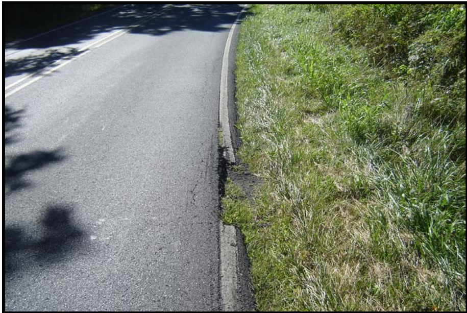
Pavement deterioration on north of Meginnes Road
