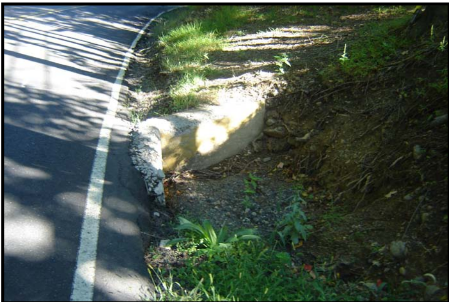
Inlet headwall is a potential hazard and clogged culvert pipe – PA 412 at Slifer Valley Road
