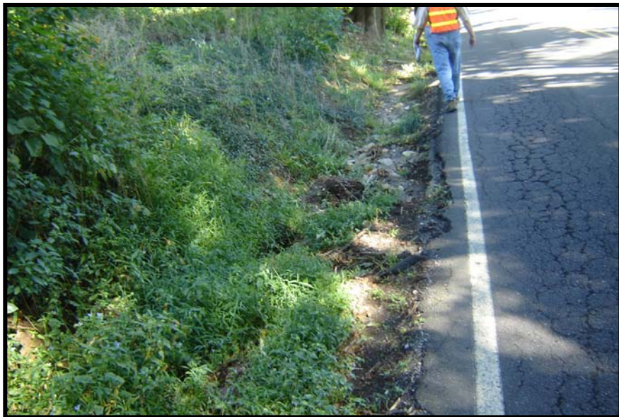
Steep drop off and edge of shoulder washed out at 3370 Main Street
