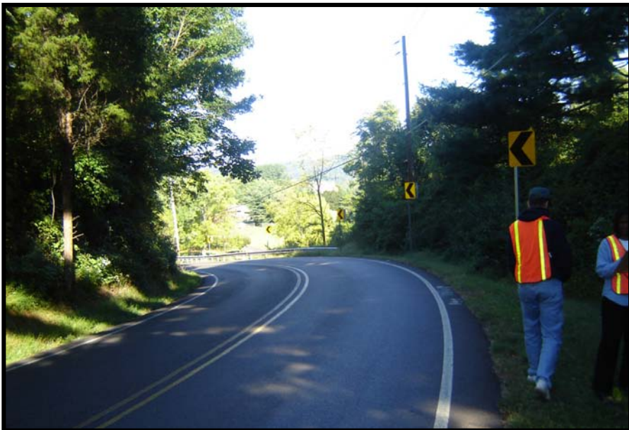
Guide rail appears too low in the vicinity of Bodder Road
