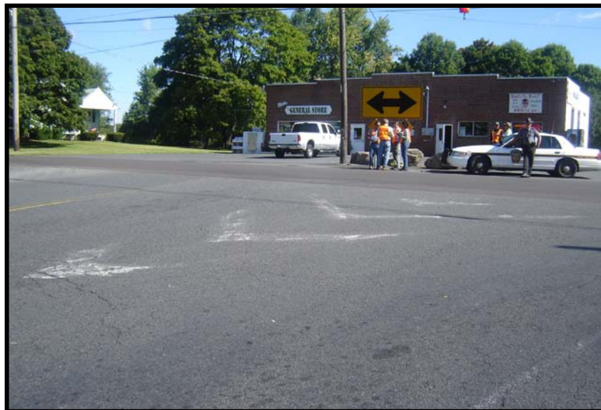
Mountain View Drive looking northbound pavement markings have faded
