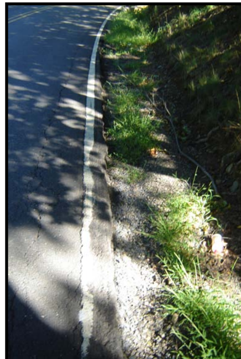
Drop off on the inside of curve – PA 412 at Slifer Valley Road
