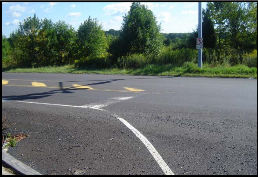
Pavement markings faded at PA 611/PA 412 intersection
