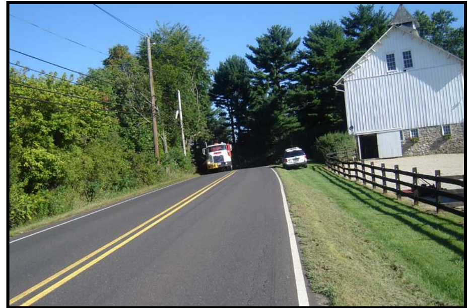
Northbound lane prior to curve has an excessive cross slope and roadway is failing.
