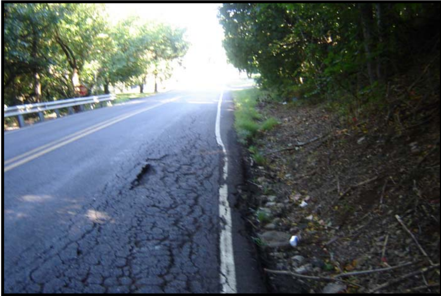
Pavement deterioration on PA 412 at Slifer Valley Road
