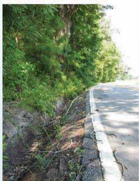
PHOTO SHOWS THE LACK OF A PAVED SHOULDER AND CLOSE PROXIMITY OF FIXED OBJECTS TO THE ROADWAY.
