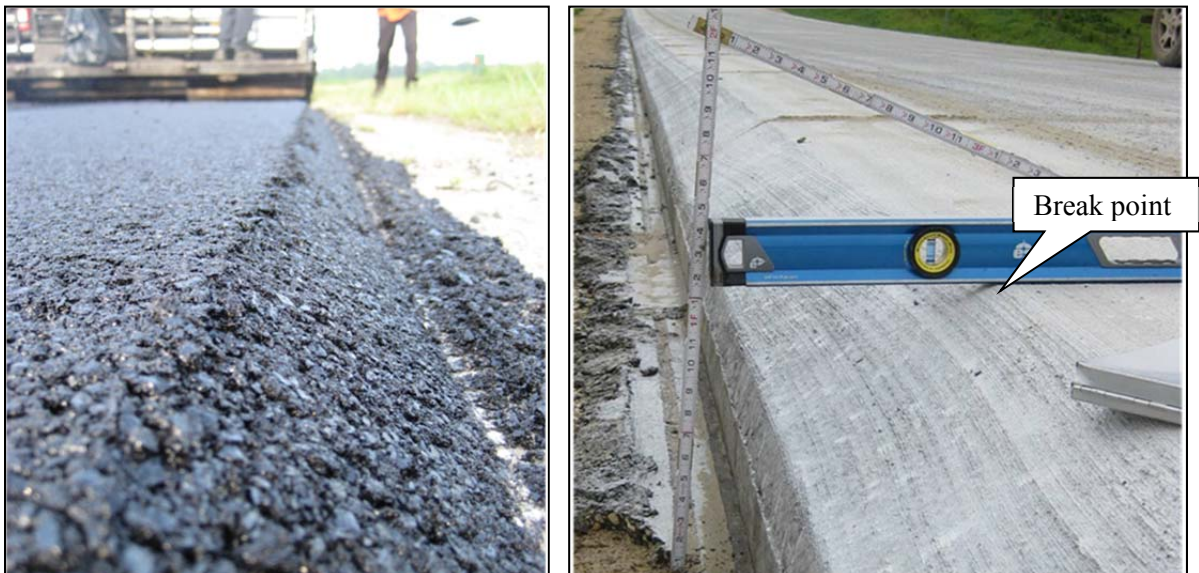
(a) AC Project.
