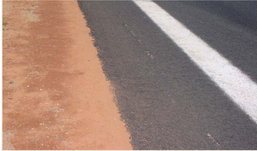
Figure 8. Safety Edge SM completely covered by shoulder backing material.
