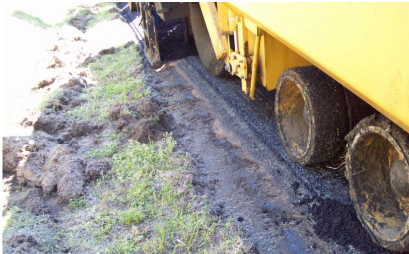
Figure 9. Paver positioned to align the Safety Edge SM break point over the existing pavement.
