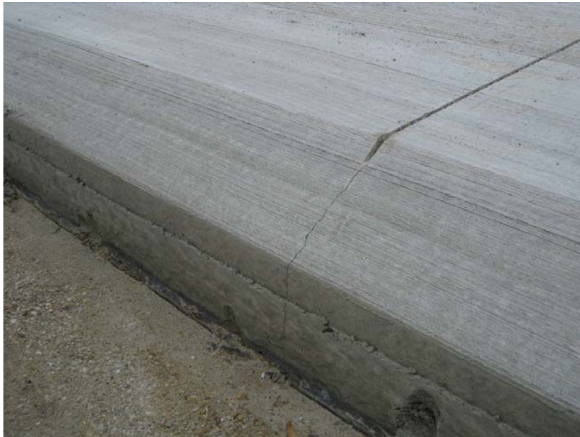
Figure 16. Sawcut and crack at the formed joint on one of the Safety Edge SM demonstration projects.
