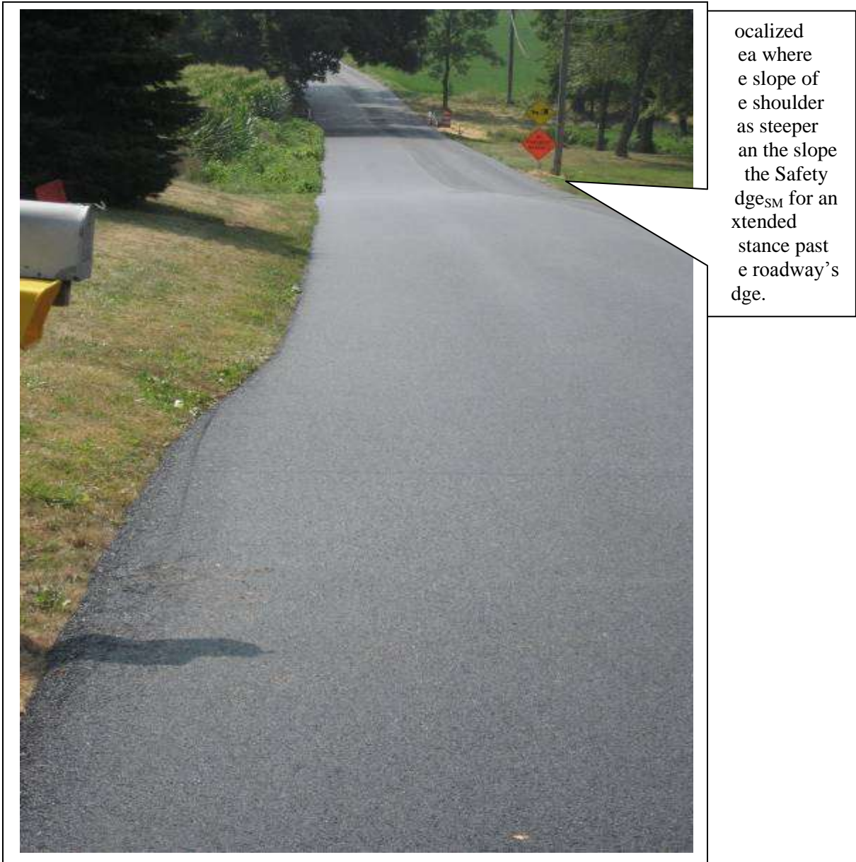
Figure 19. Area where the slope of the shoulder was steeper than the Safety Edge SM slope.
