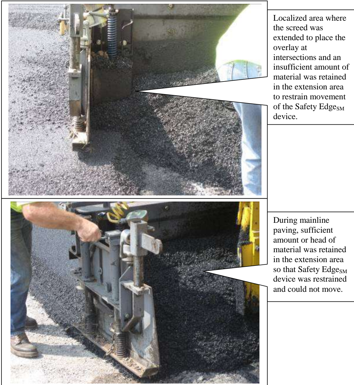
Figure 20. Photographs showing where a sufficient and insufficient amount of head of HMA was retained in the extended auger chamber area.
