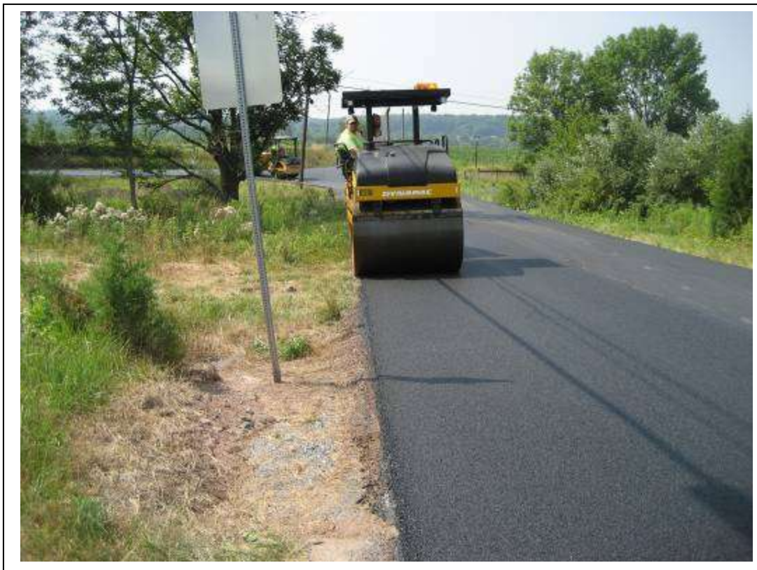
Figure 22. Vibratory steel wheel roller used in the breakdown position shown compacting the Safety Edge SM – first pass overhung the edge about 4 inches.
