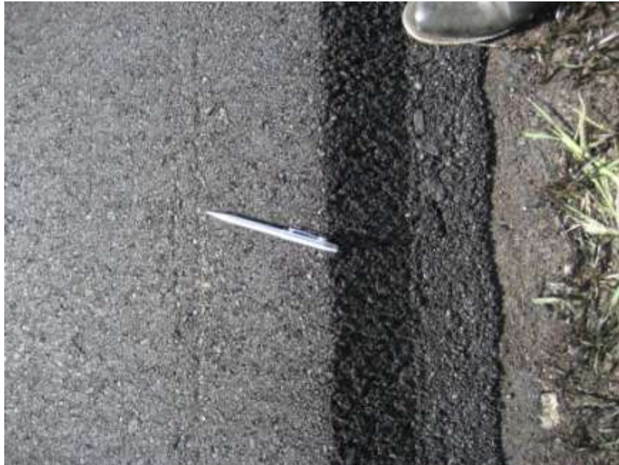
Figure 22. Longitudinal mark left by delaying the breakdown rolling of the Safety Edge SM ; image taken after finish rolling.
