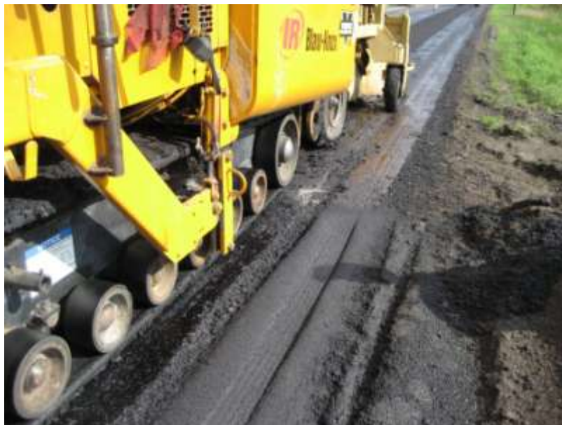
Figure 5. Close-up of the full-depth patch area with surface depressions from the belly-dump trucks and paver.
