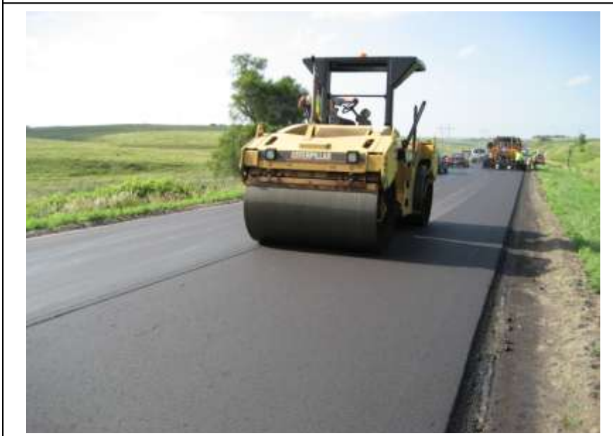
(b) Second pass of Caterpillar breakdown roller in vibratory mode along the hot-side of the longitudinal joint.
