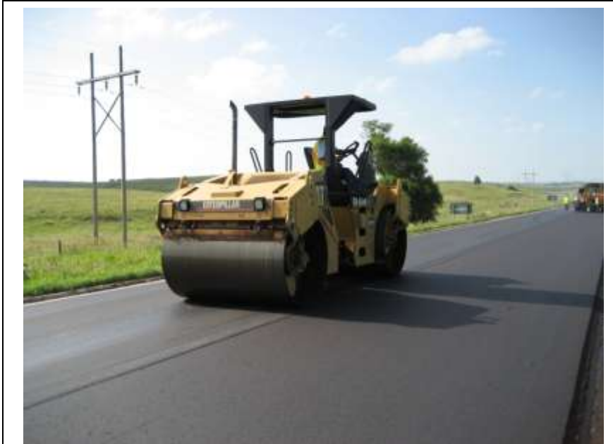
(a) First pass of Caterpillar breakdown roller in static mode along the cold-side of the longitudinal joint.
