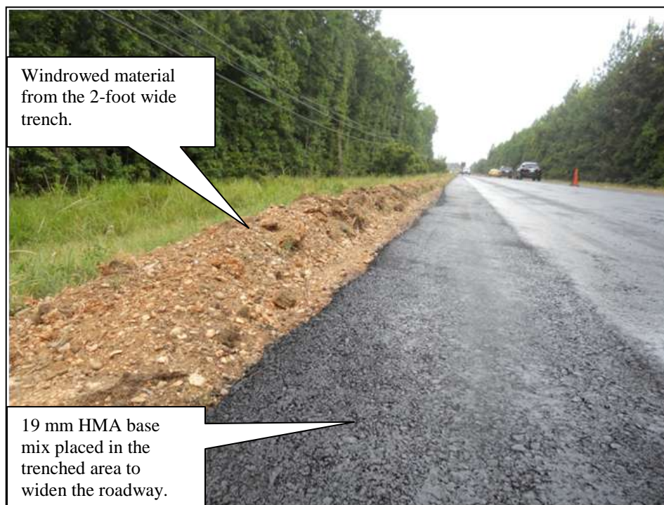
Figure 5. General view of the 19 mm HMA base placed to widen the roadway.
