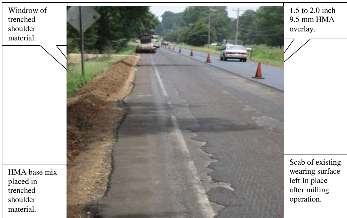
Figure 4. General overview of the existing HMA pavement after milling; minor distressed area (view is towards the east).
