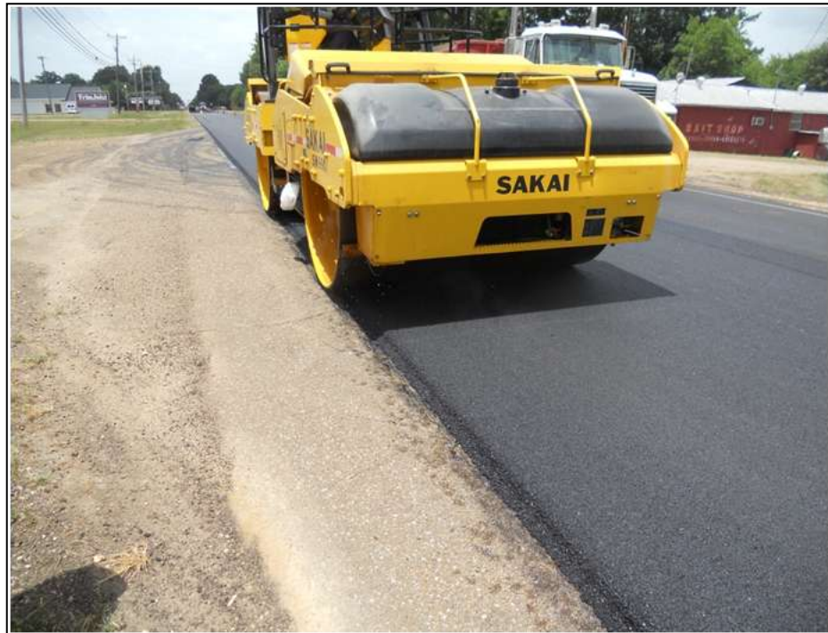
(a) First pass of Sakai roller is 4 to 6 inches over the edge of the mat.
