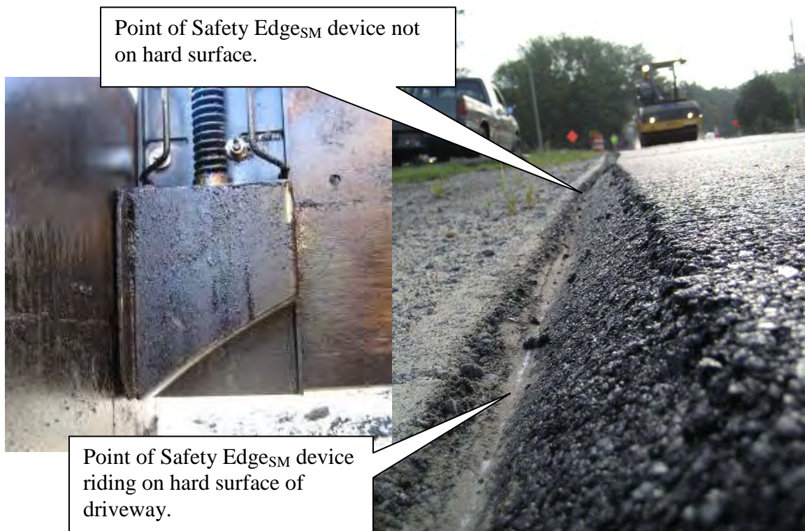
Figure 18. Point of Safety Edge SM scratching the surface of an intersecting driveway.
