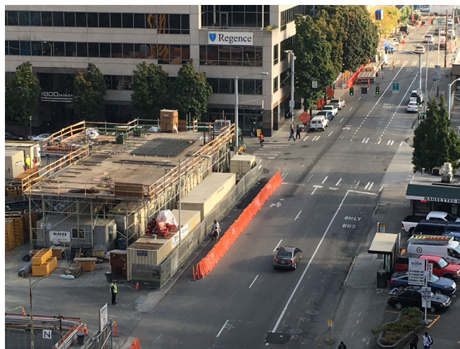
To meet the needs of all road users and ensure connections during construction, agencies can set policies that establish safe and continuous routes around work zones. Credit: Dan Gelinne, PBIC Image Library.
