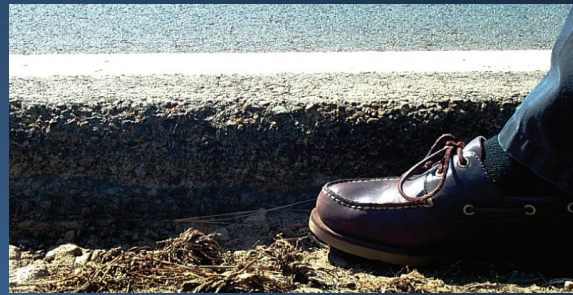
Sharp, steep pavement edge drop-offs can contribute to crashes.
