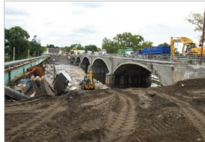
One impacted project was the Bridge Avenue Bridge Project in Cohoes, NY
