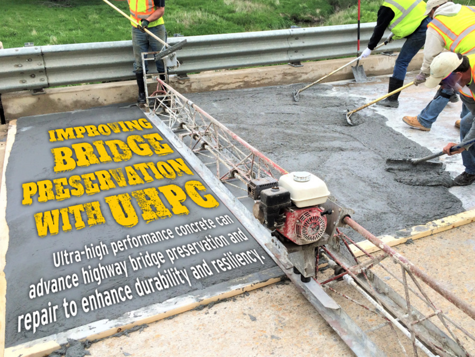
Ultra-high performance concrete (UHPC) has long been used for new construction in connections between prefabricated bridge elements. In the last few years, its use in bridge repair and preservation has increased as well. Here, crews install the first U.S. deployment of UHPC as a bridge deck overlay on a reinforced concrete slab bridge located in Brandon, IA, completed in May 2016.
