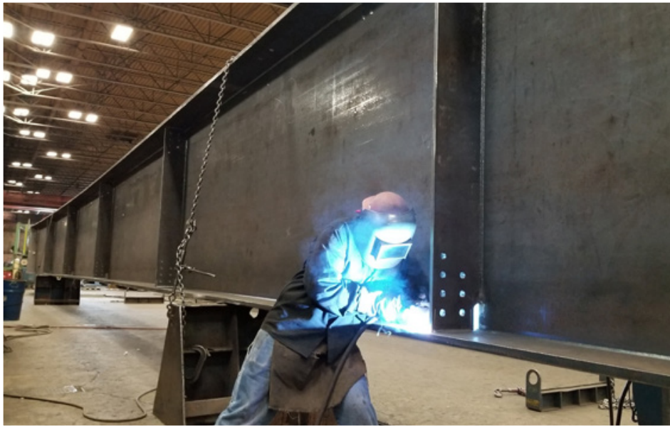
The welds between steel plates used in fabricating bridge girders can develop flaws both during manufacturing and after construction.
