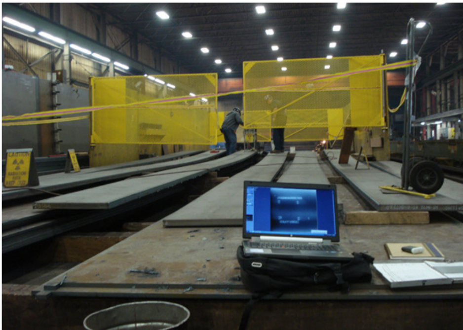
Radiation boundaries in a fabrication shop help keep workers safe from the high levels of radiation needed to radiographically inspect welds.
