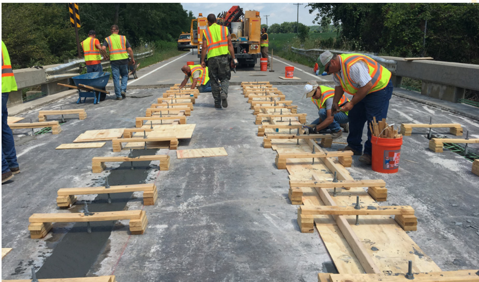
In 2017, the St. Clair County Road Commission in Michigan was the first to deploy an open-source UHPC mixture on a U.S. bridge. UHPC was used to repair the joints between the bridge's precast double T-beams.
