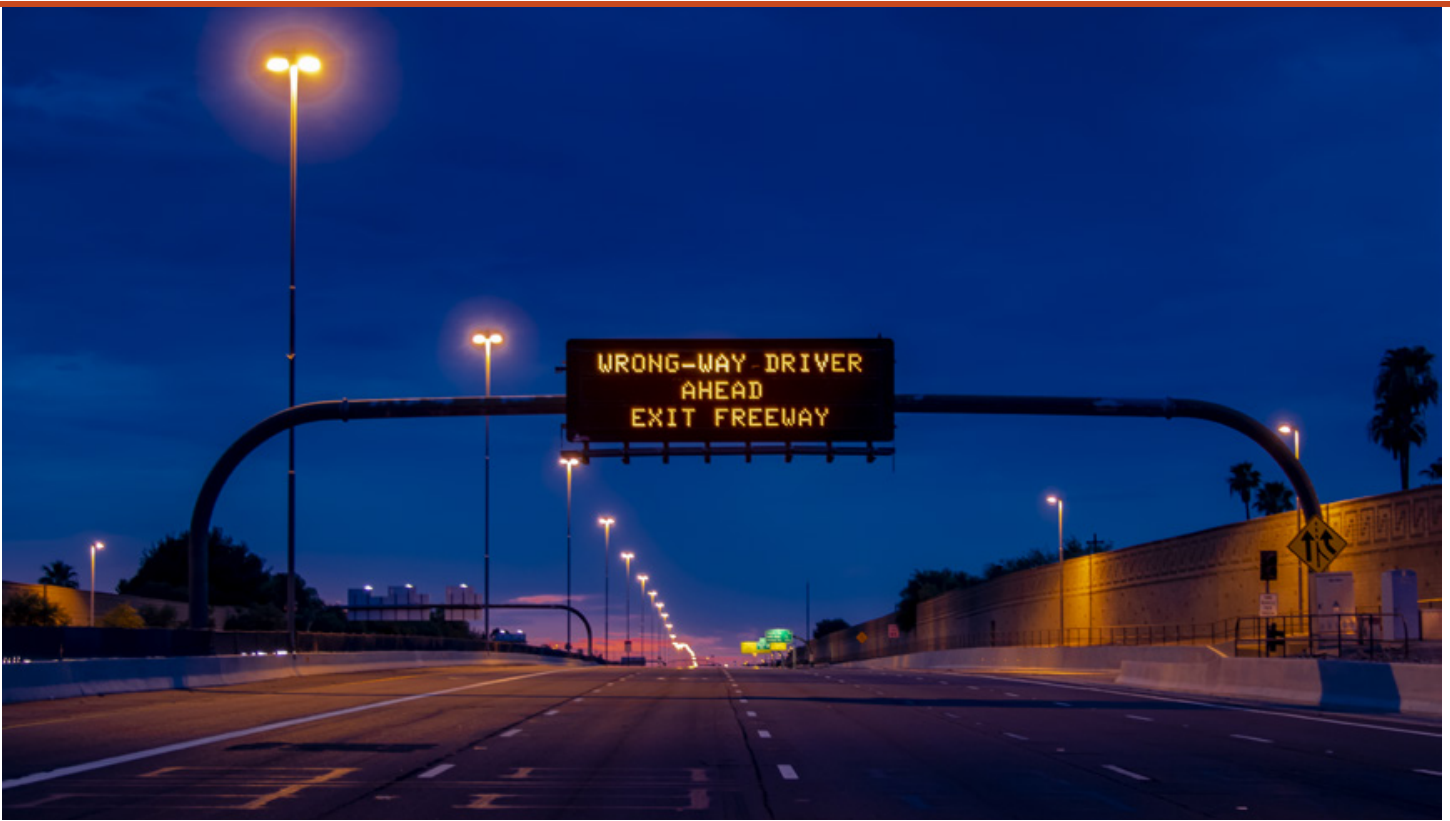
Overhead changeable message signs warn other drivers about wrong-way drivers on the freeway as part of Arizona's pilot project.
