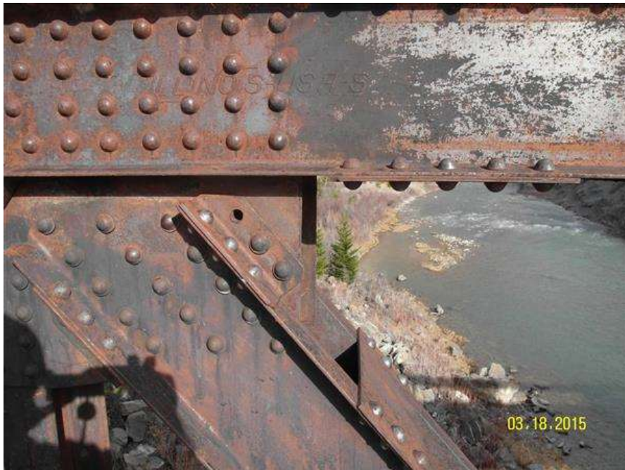
PHOTO #2 MTA-SR-001, SUN RIVER BRIDGE, PHOTO BY GARY GRASSEL. VIEW OF A MISSING FASTENER AT THE UPSTREAM SIDE, RIGHT TRUSS, FIRST TOP JOINT FROM THE RIGHT BEARING. (03/18/2015)
