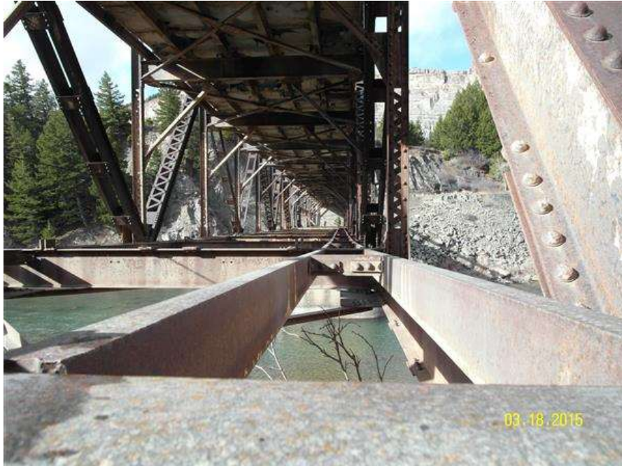
PHOTO #7 MTA-SR-001, SUN RIVER BRIDGE, PHOTO BY GARY GRASSEL. THIS PHOTO IS A VIEW LOOKING FROM THE LEFT ABUTMENT TO THE CENTER PIER ON THE UPSTREAM SIDE OF THE BRIDGE. NOTE THE SAG IN THE TRUSS APPROXIMATELY AT MID-SPAN OF THE UPSTREAM SIDE ONLY. CONNECTIONS HAVE BEEN INSPECTED BY RECLAMATION CLIMB TEAM AND NOTHING OUT OF THE NORMAL WAS OBSERVED AT THE CONNECTIONS OR MEMBERS. (03/18/2015)
