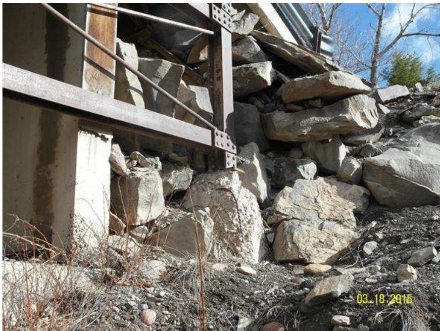
PHOTO #8 MTA-SR-001, SUN RIVER BRIDGE, PHOTO BY GARY GRASSEL. THIS IS A VIEW OF THE SUPPORT PIER ON THE LEFT DOWNSTREAM APPROACH SPAN OF THE BRIDGE. RECOMMEND REPLACING THIS EXISTING PIER WITH NEW REINFORCED CONCRETE PIER. (03/18/2015)
