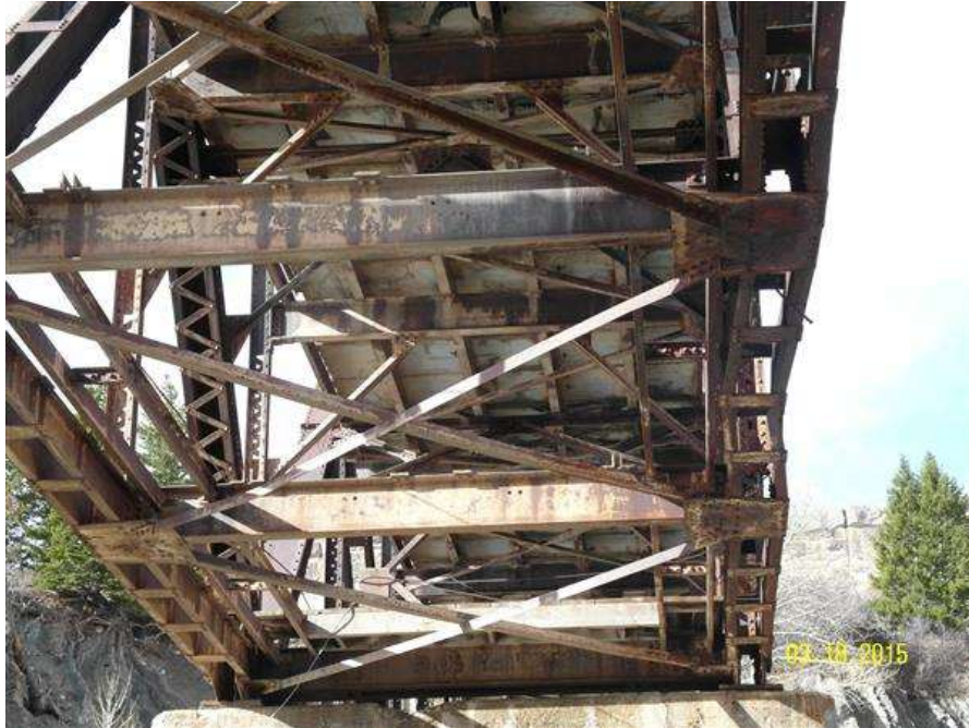
PHOTO #11 MTA-SR-001, SUN RIVER BRIDGE, PHOTO BY GARY GRASSEL. THIS PHOTO SHOWS THE BOTTOM CORD OF THE LEFT UPSTREAM TRUSS. THE BENT LOWER CORD HAS BEEN INSPECTED BY THE RECLAMATION CLIMB TEAM AND NOTHING WAS OBSERVED TO BE IN NEED OF REPAIR. (03/18/2015)
