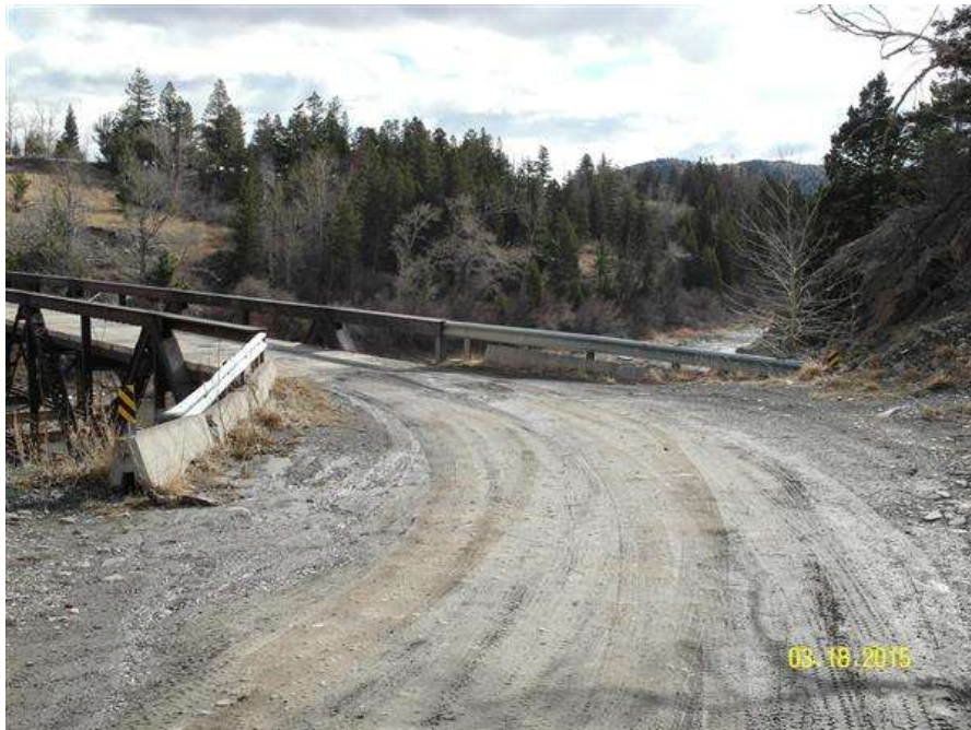
PHOTO #6 MTA-SR-001, SUN RIVER BRIDGE, PHOTO BY GARY GRASSEL. THIS IS A VIEW OF THE RIGHT APPROACH TO THE BRIDGE. (03/18/2015)
