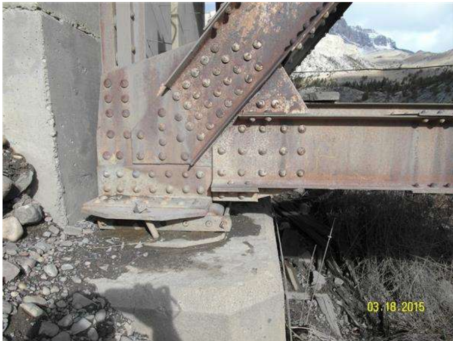
PHOTO #12 MTA-SR-001, SUN RIVER BRIDGE, PHOTO BY GARY GRASSEL. THIS IS A VIEW OF THE BEARING ASSEMBLY ON THE DOWNSTREAM SIDE OF THE RIGHT TRUSS AND RIGHT APPROACH. NOTE TRUSS ANCHOR BOLT IS BENT AND TRUSS BEARING PLATE COMING OFF THE ROLLERS. (03/18/2015)
