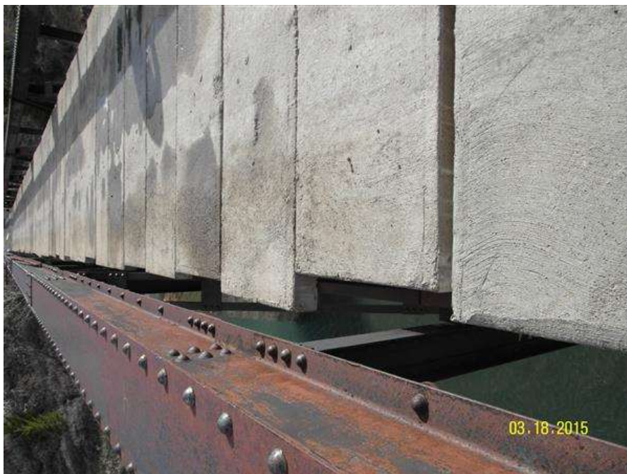
PHOTO #4 MTA-SR-001, SUN RIVER BRIDGE, PHOTO BY GARY GRASSEL. THIS PHOTO IS A VIEW PARALLEL TO BRIDGE CENTER LINE LOOKING AT THE DOWNSTREAM SIDE OF THE BRIDGE SURFACE. THE PRECAST PLANKS HAVE SHIFTED UPSTREAM AND DOWNSTREAM. RECOMMEND ALL PANELS ARE ATTACHED TO BEAMS AND ADJACENT PANELS TO CREATE NECESSARY DIAPHRAGM. (03/18/2015)
