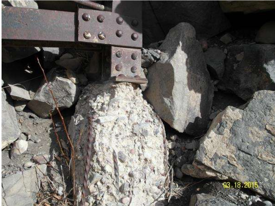
PHOTO #9 MTA-SR-001, SUN RIVER BRIDGE, PHOTO BY GARY GRASSEL. THIS PHOTO IS A CLOSER VIEW OF THE PIER IN PHOTO # 8. (03/18/2015)
