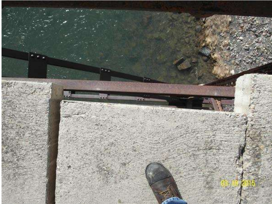
PHOTO #3 MTA-SR-001, SUN RIVER BRIDGE, PHOTO BY GARY GRASSEL. THIS PHOTO SHOWS THAT THE PRECAST FLOOR PLANKS ARE NOT FASTENED TO THE SUPERSTRUCTURE BEAM MEMBERS. PLANKS CAN MOVE UPSTREAM OR DOWNSTREAM AND MAY SHIFT A DISTANCE WHERE THEIR USE AS A TRAFFIC SURFACE WILL BE A CRITICAL FAILURE MODE. (03/18/2015)
